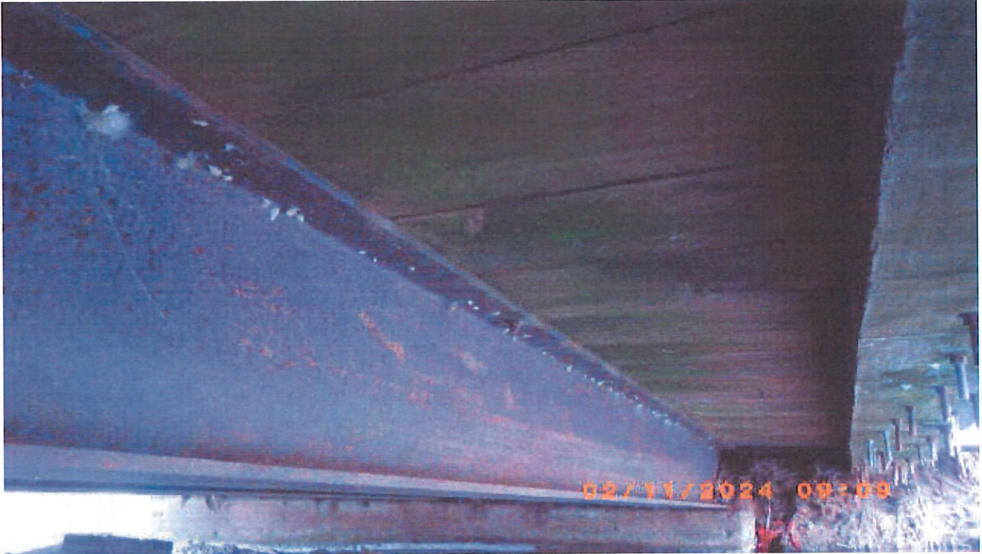
Typical underside of deck / green mold
