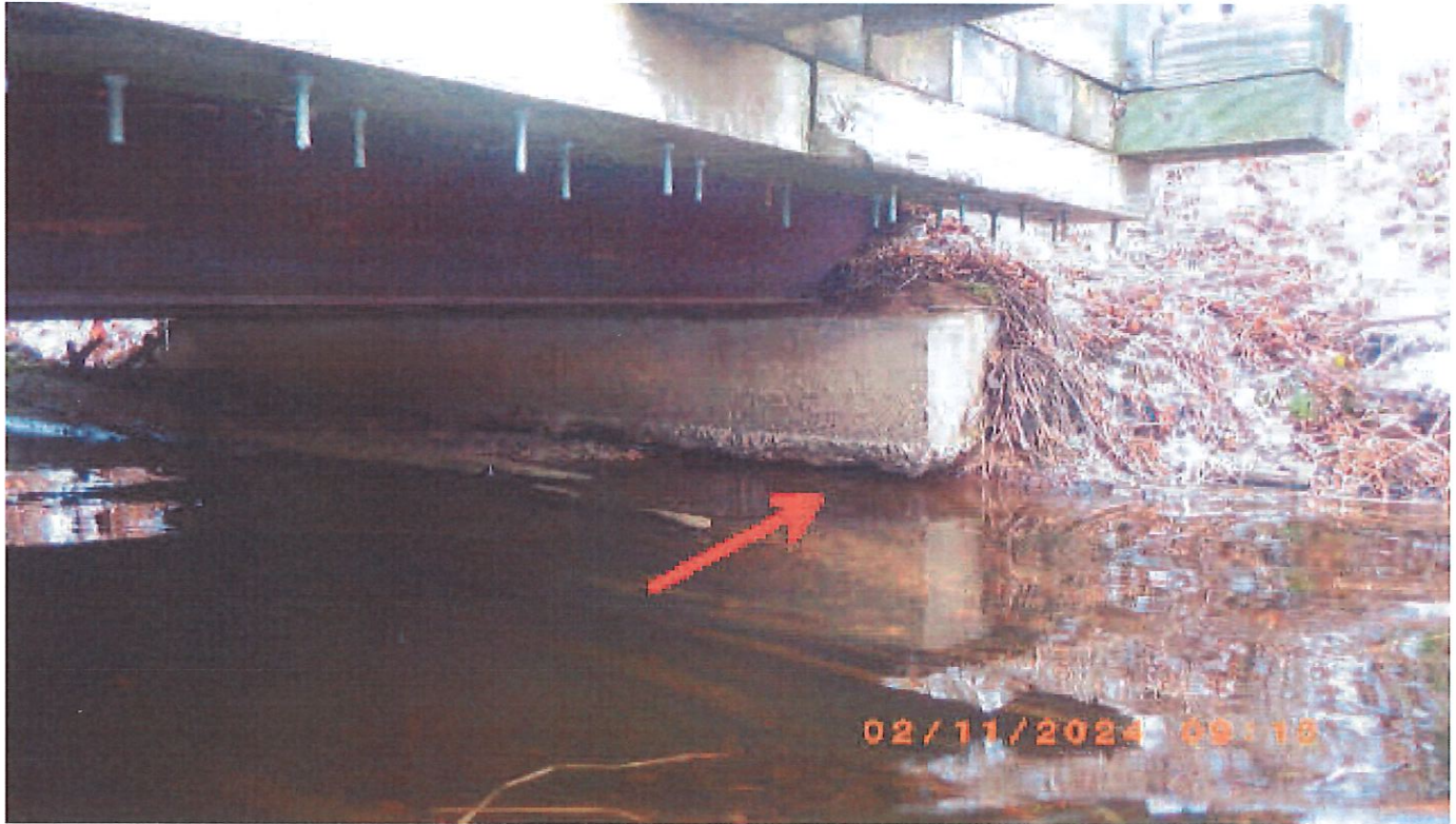
East sill undermined up to 12" deep at south end
