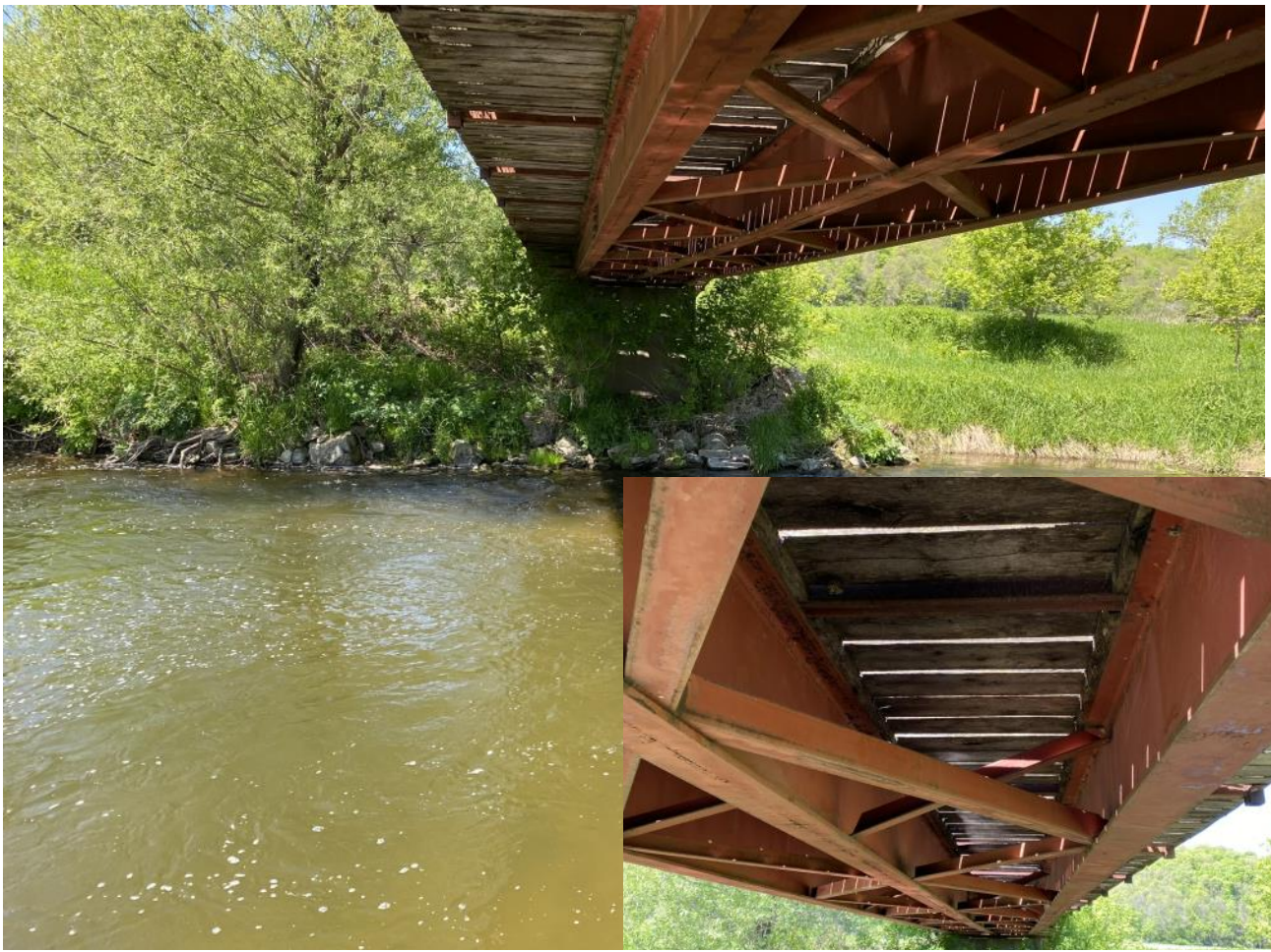
Though appears to be well built it still wiggles under a light load. Welds don't appear as strong as they should
