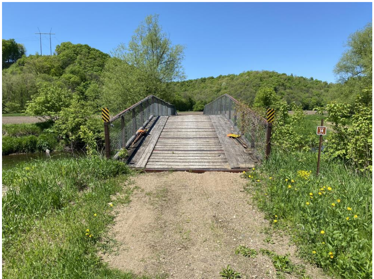
Approach from the south. Groomers are unable to cross this bridge and take a river crossing instead.
