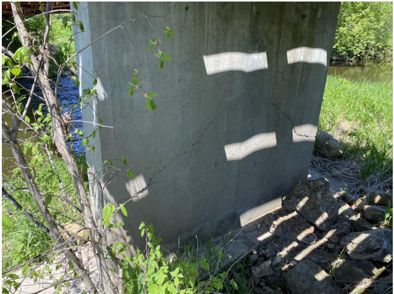
Not sure if this is just a pour line or a crack in the abutment
