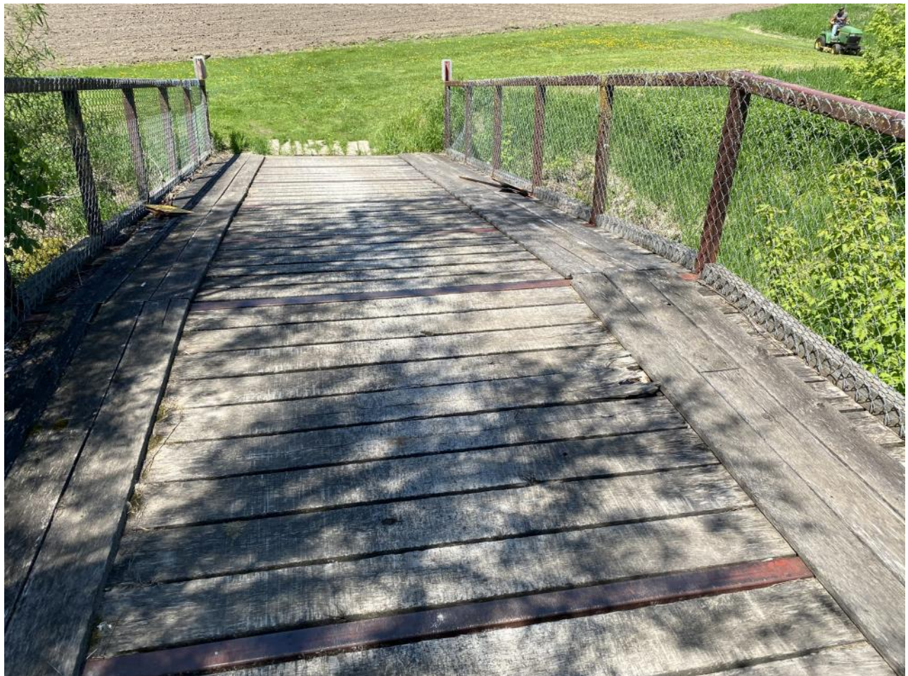
The riding lawn mower in the upper right corner made the bridge wiggle when crossing (Landowner)
