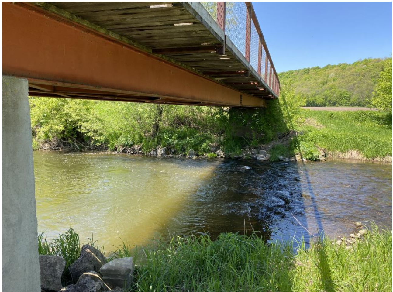
The area is in need of more rip rap to protect the bridge
