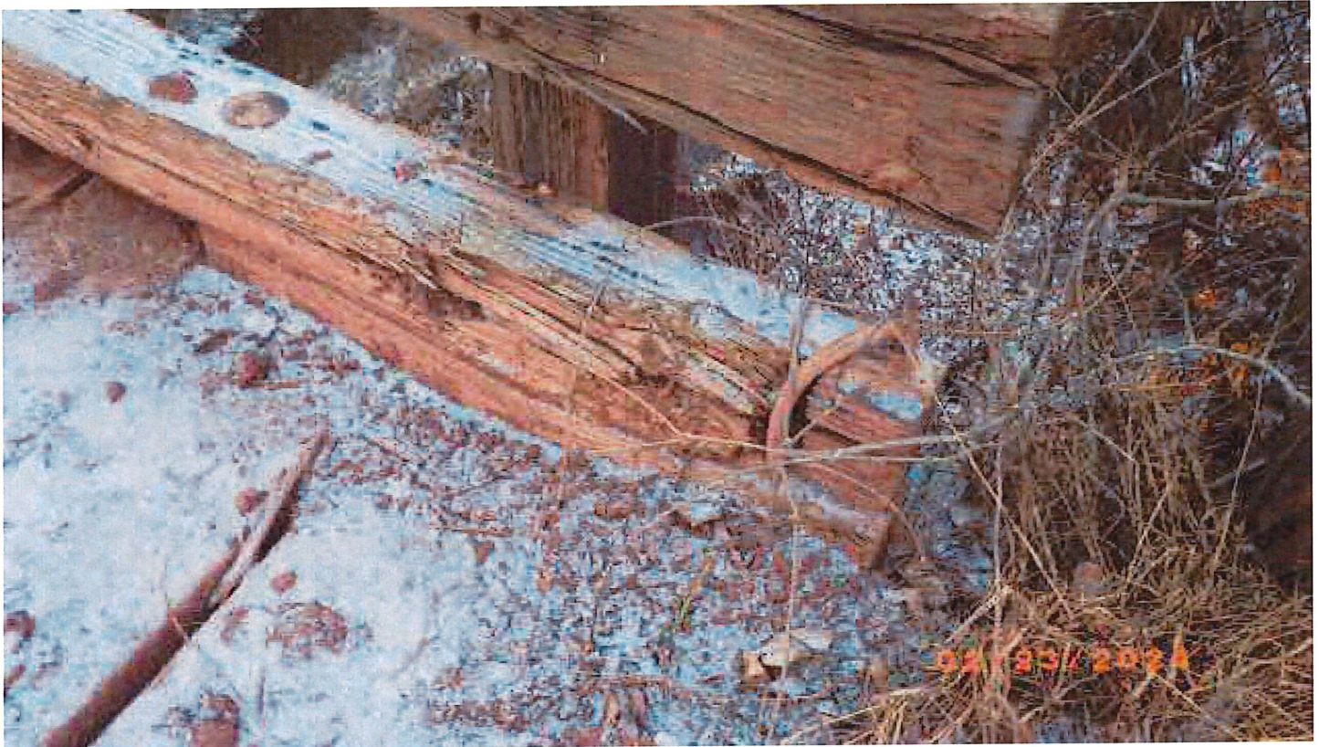
Damaged curb end, North side.
