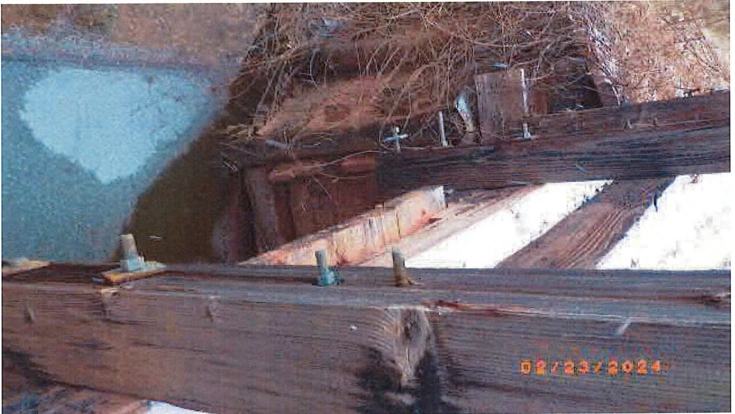
Missing rail hardware
