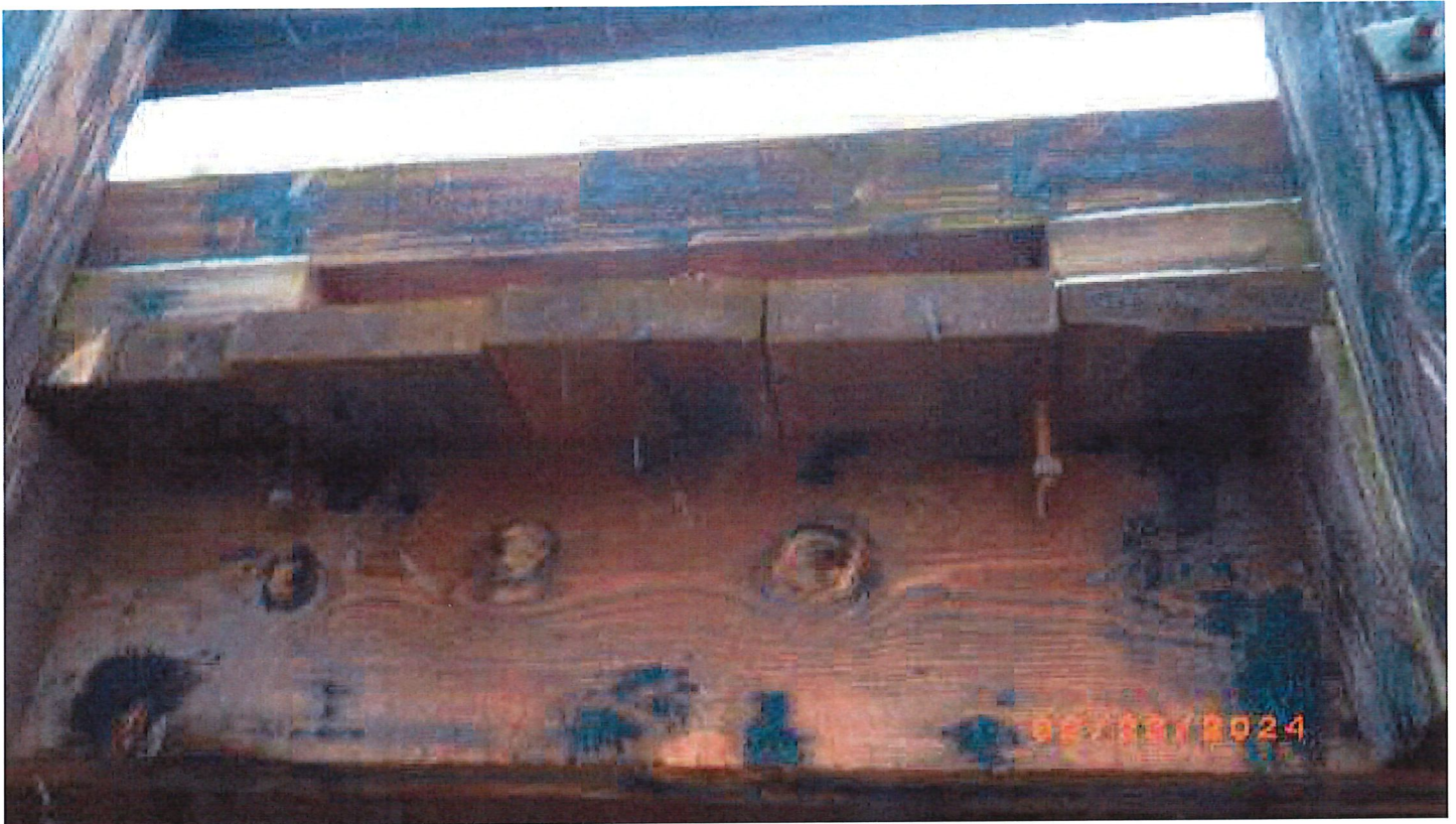
Curb bolts loose.
