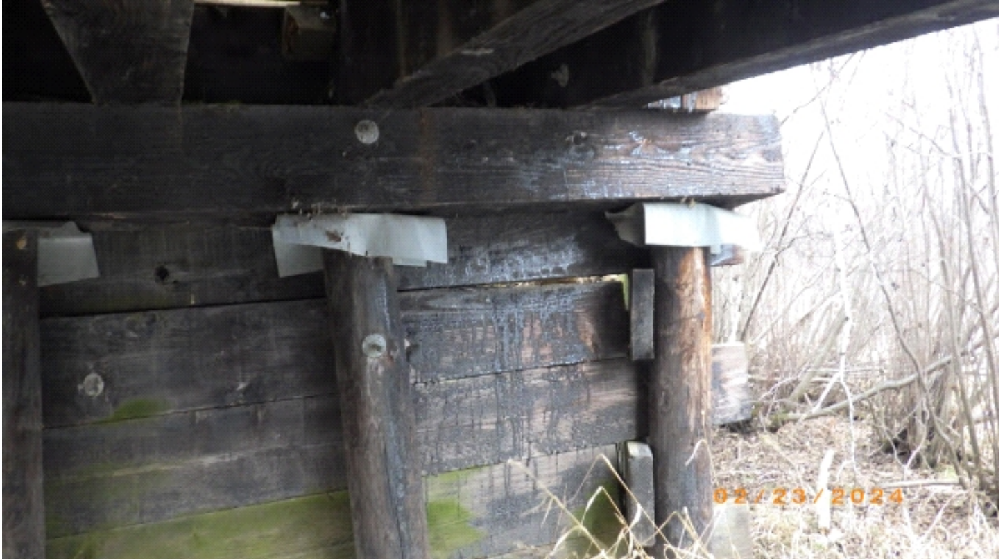
Gaps in backing boards and gaps between the cap and piles.
