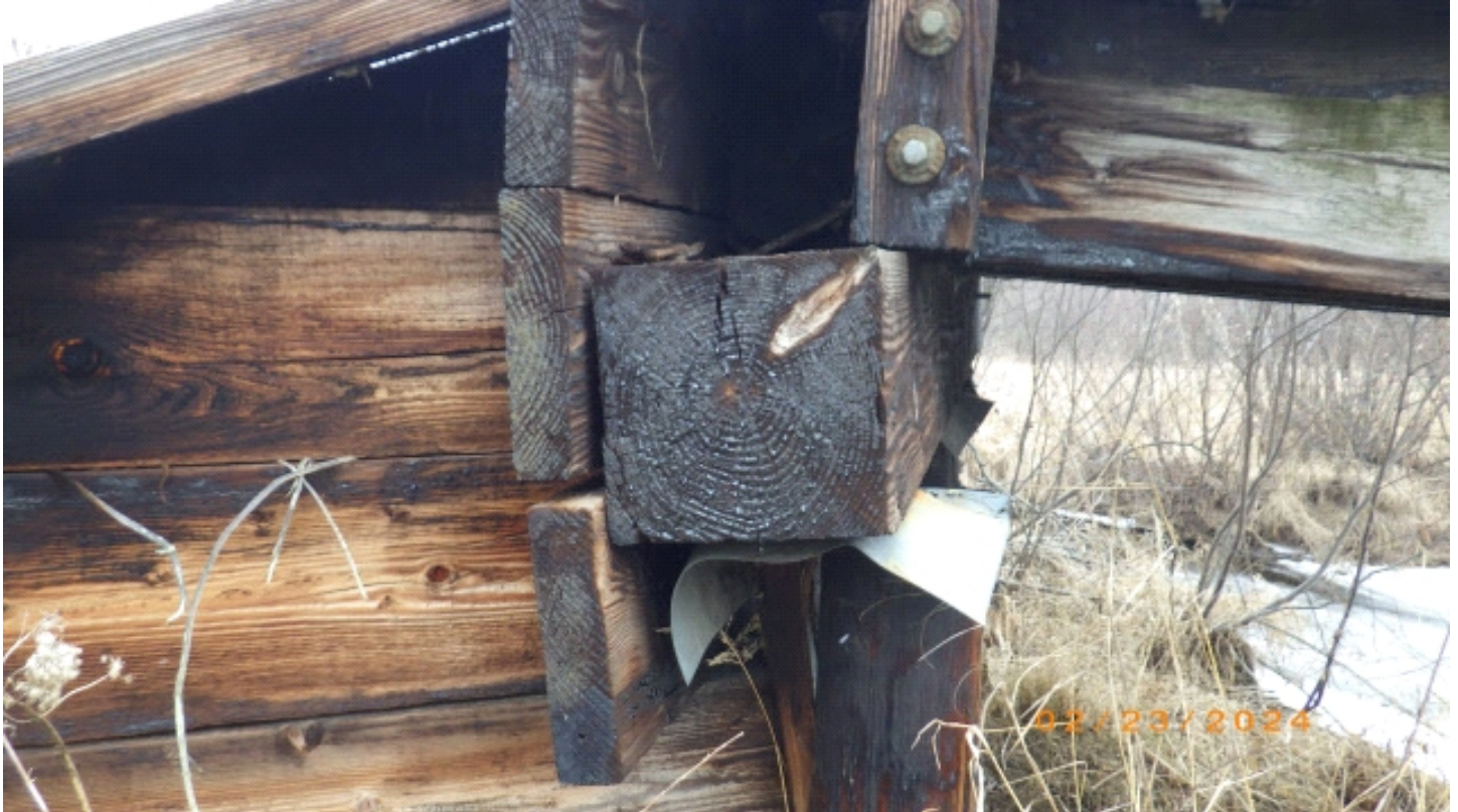
Pile cap pushed of the piles.
