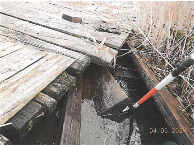
Loose and Missing Timber Supports in the Southeast Quadrant
