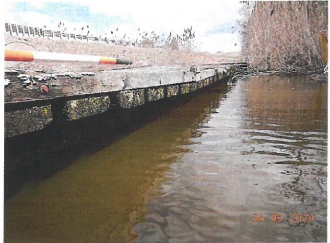
Sag in Main Span
