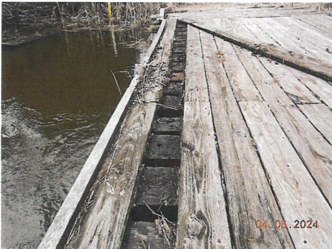
Main Span – Wearing Deck Board Removed Showing Minor to Moderate Rotten Transverse Boards
