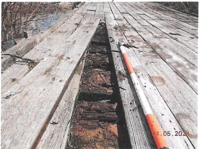
Typical Surface Rot of Transverse Deck Boards
