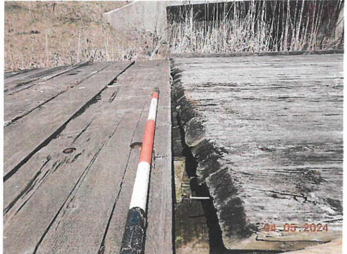
Gap Between Approach Span and Main Span (West Shown)
