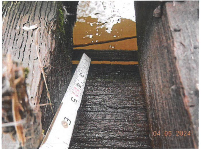
South Fascia Timber Girder (Pole) with Minor Splinter and Section Loss
