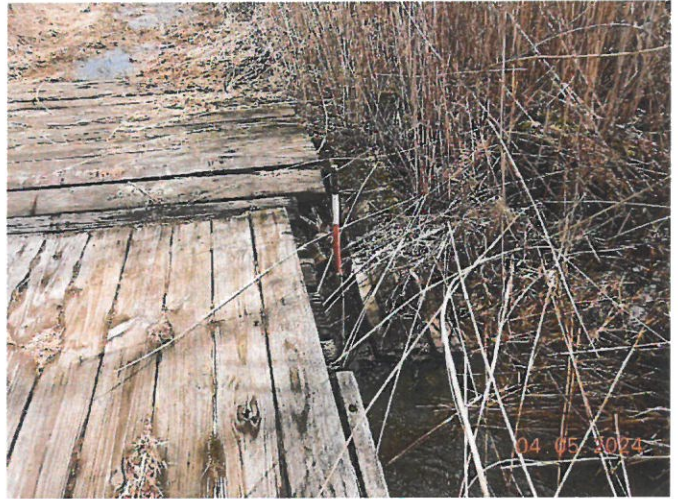
Southeast Quadrant with no Support of the Main Span
