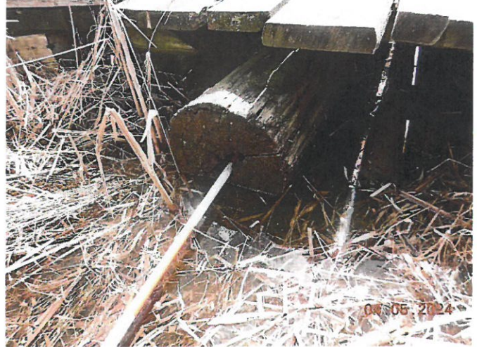
West Bank Timber Pier Log with 100% Section Loss of the Center with 14 inches of Penetration
