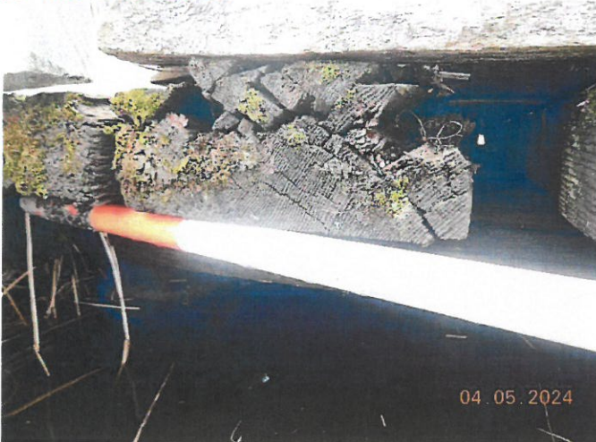
Typical Deterioration of the Transverse Deck Board Ends
