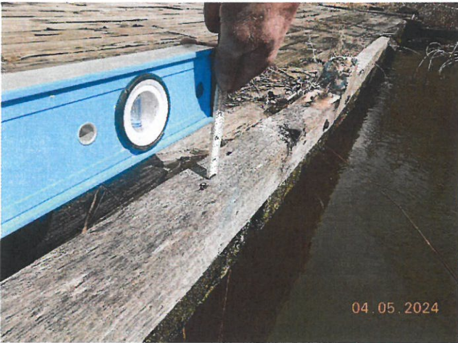
2.5 Inch Sag over 4 Feet
