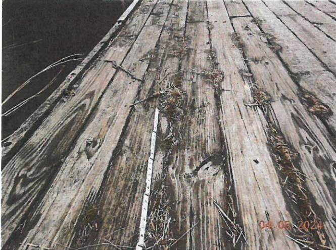
Typical Vegetation Growth in between Deck Boards
