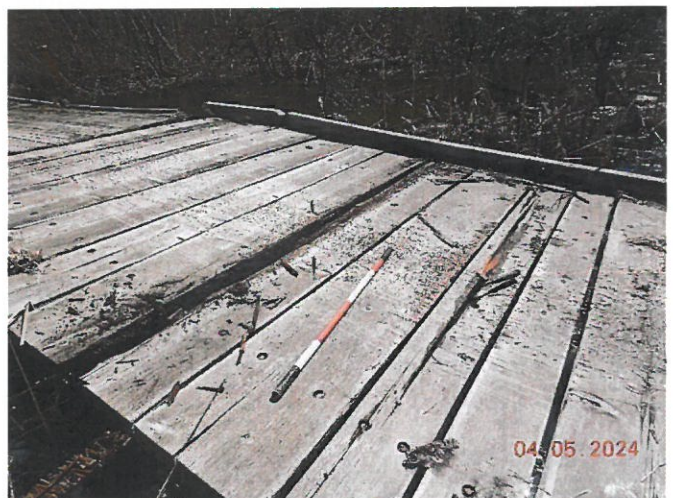
West Approach Span – Overview of Rotten Deck Boards
