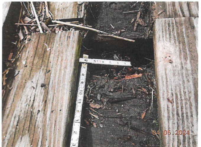
Typical Surface Rot of Transverse Deck Boards
