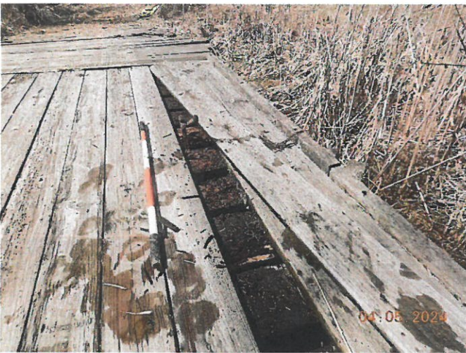
Main Span – Wearing Deck Board Removed Showing Minor to Moderate Rotten Transverse Boards
