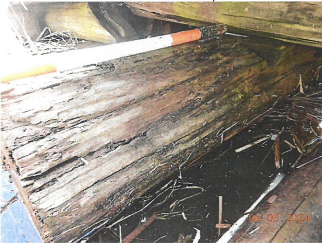
West Bank Timber Pier Log with Moderate Surface Rot and Deterioration
