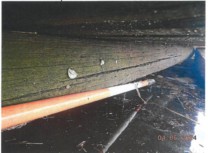
Typical Checks and Surface Rot of Timber Girders (Poles).
