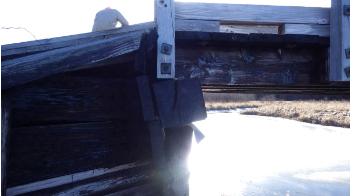
East end of south pile cap split through and severe tilt backwards
