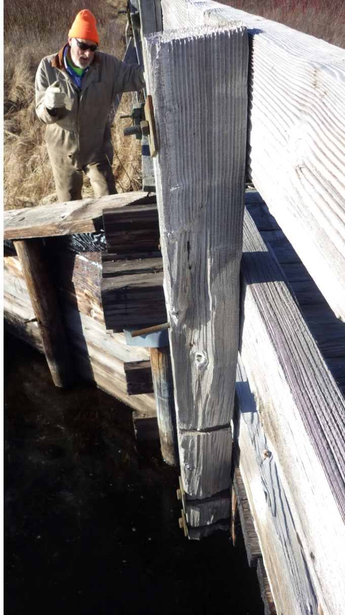
Broken rail post, upstream side
