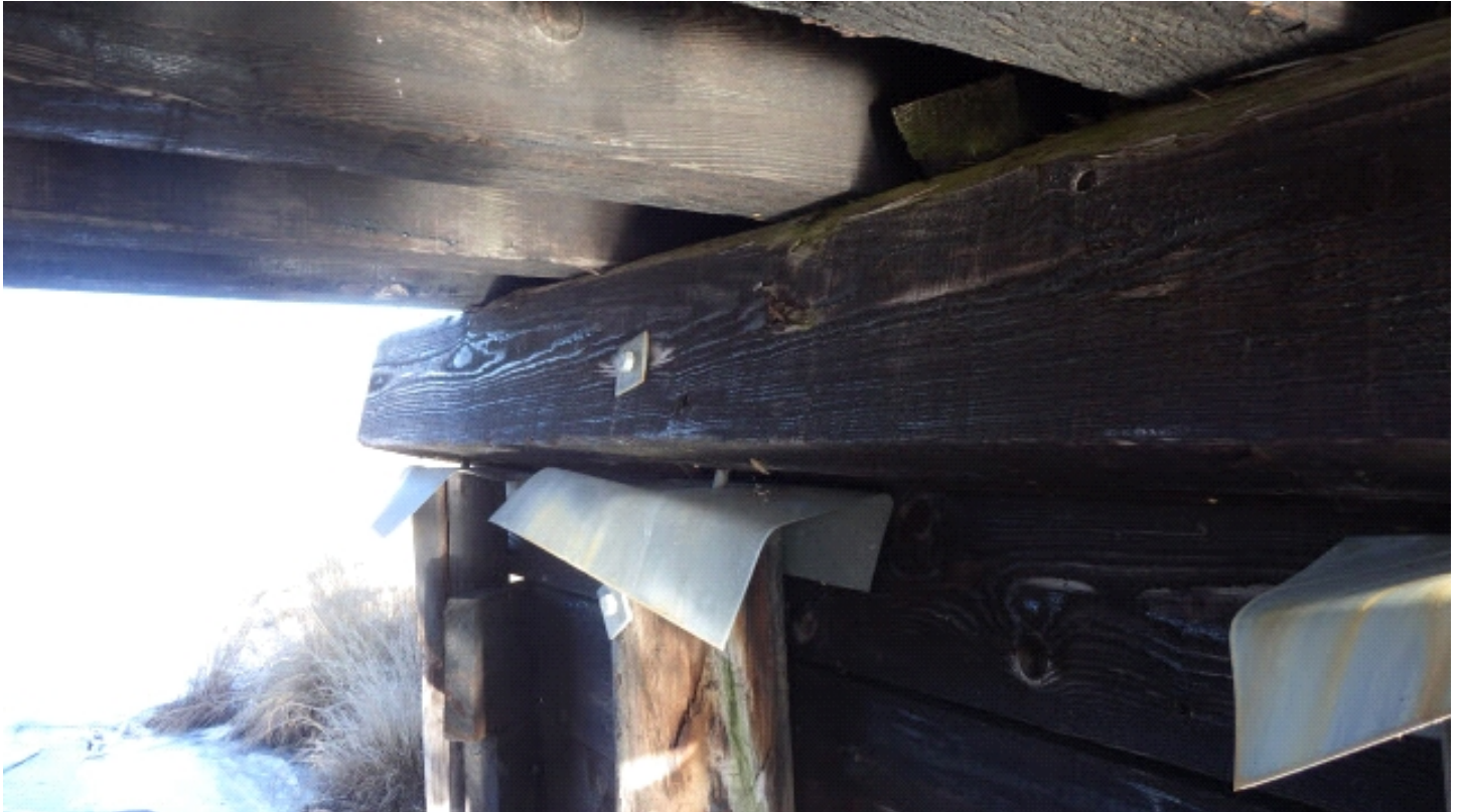
South pile cap no bearing on piles
