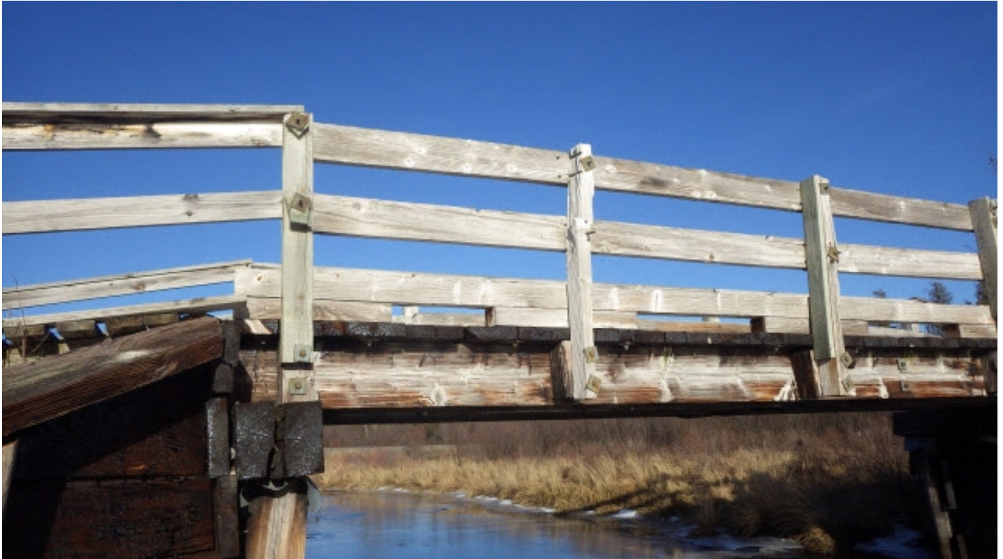
Broken rail posts, upstream side
