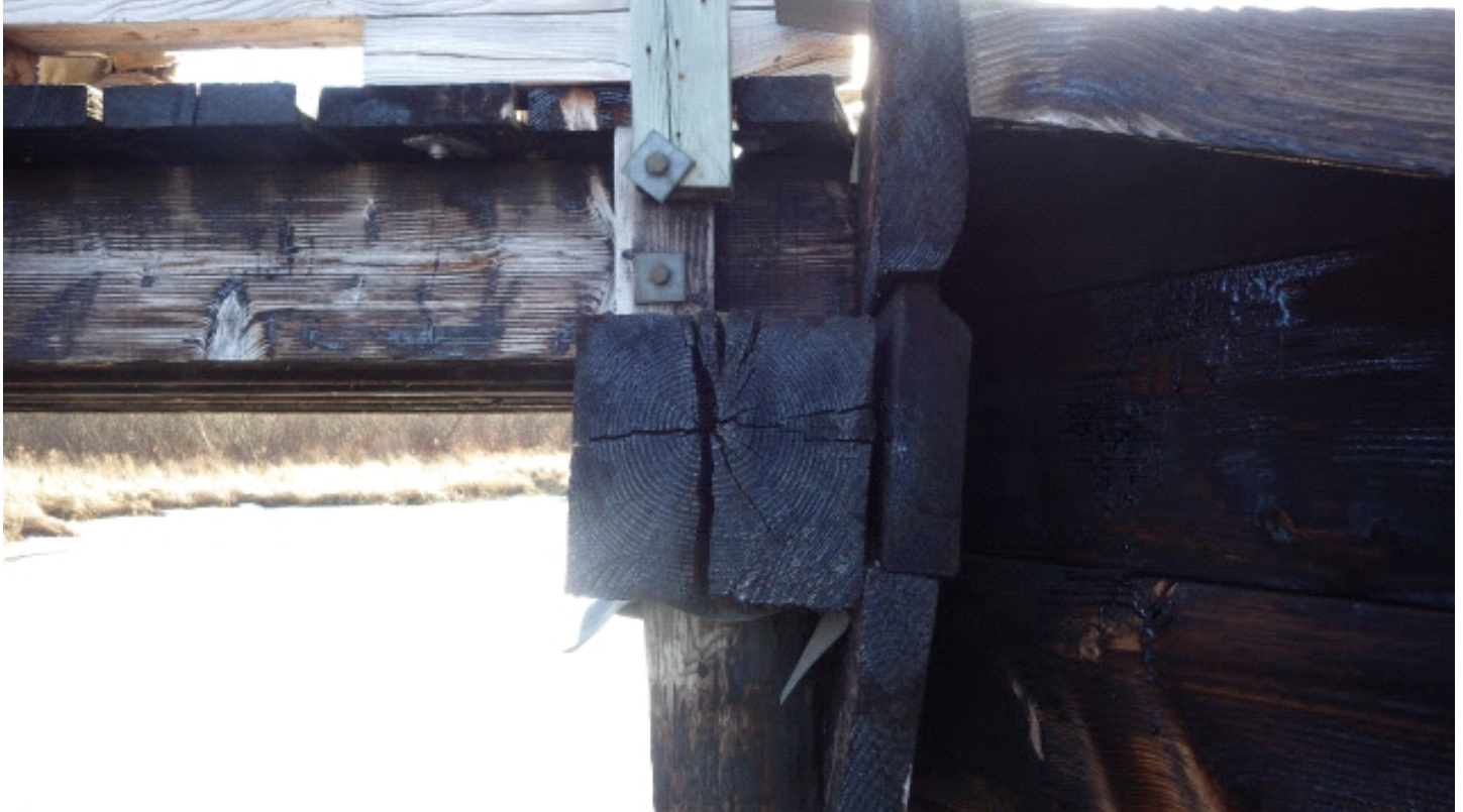
East end of north pile cap split through and moderate tilt backwards
