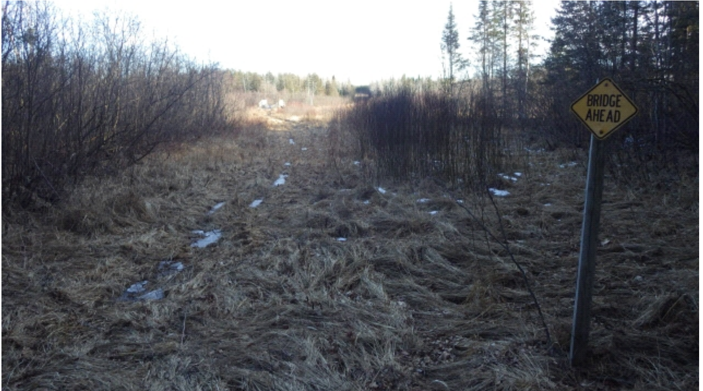
North bridge ahead sign, fair condition.
