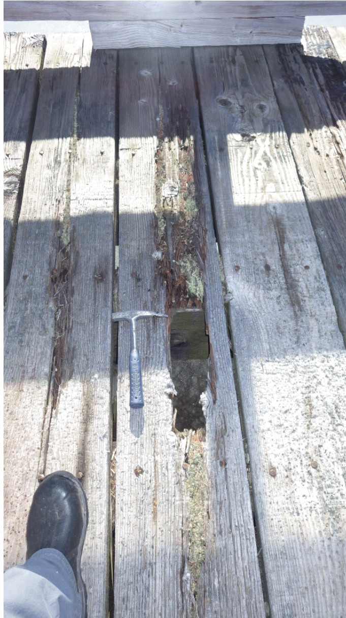
Large holes in deck
