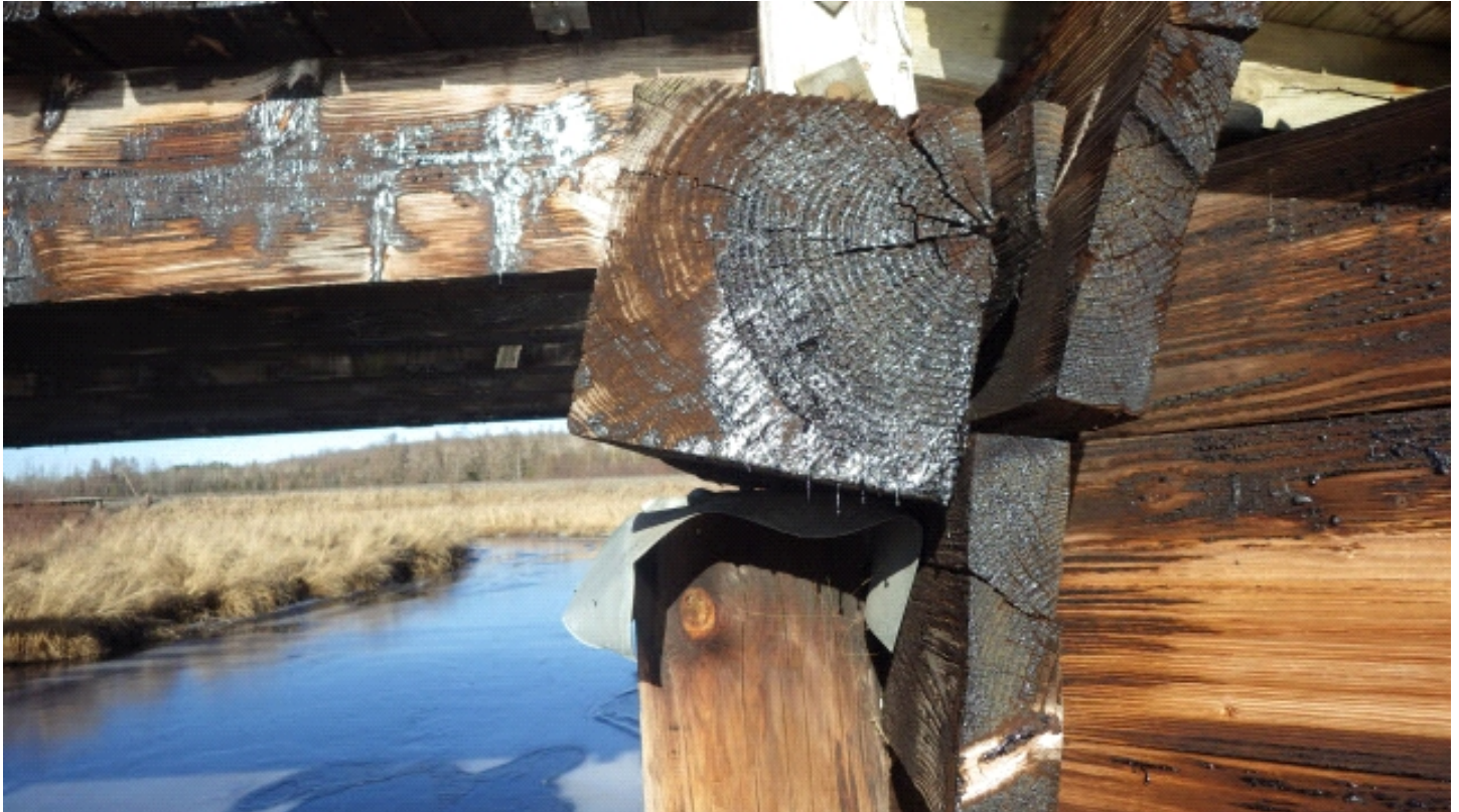
West end of south pile cap, severe tilt backwards
