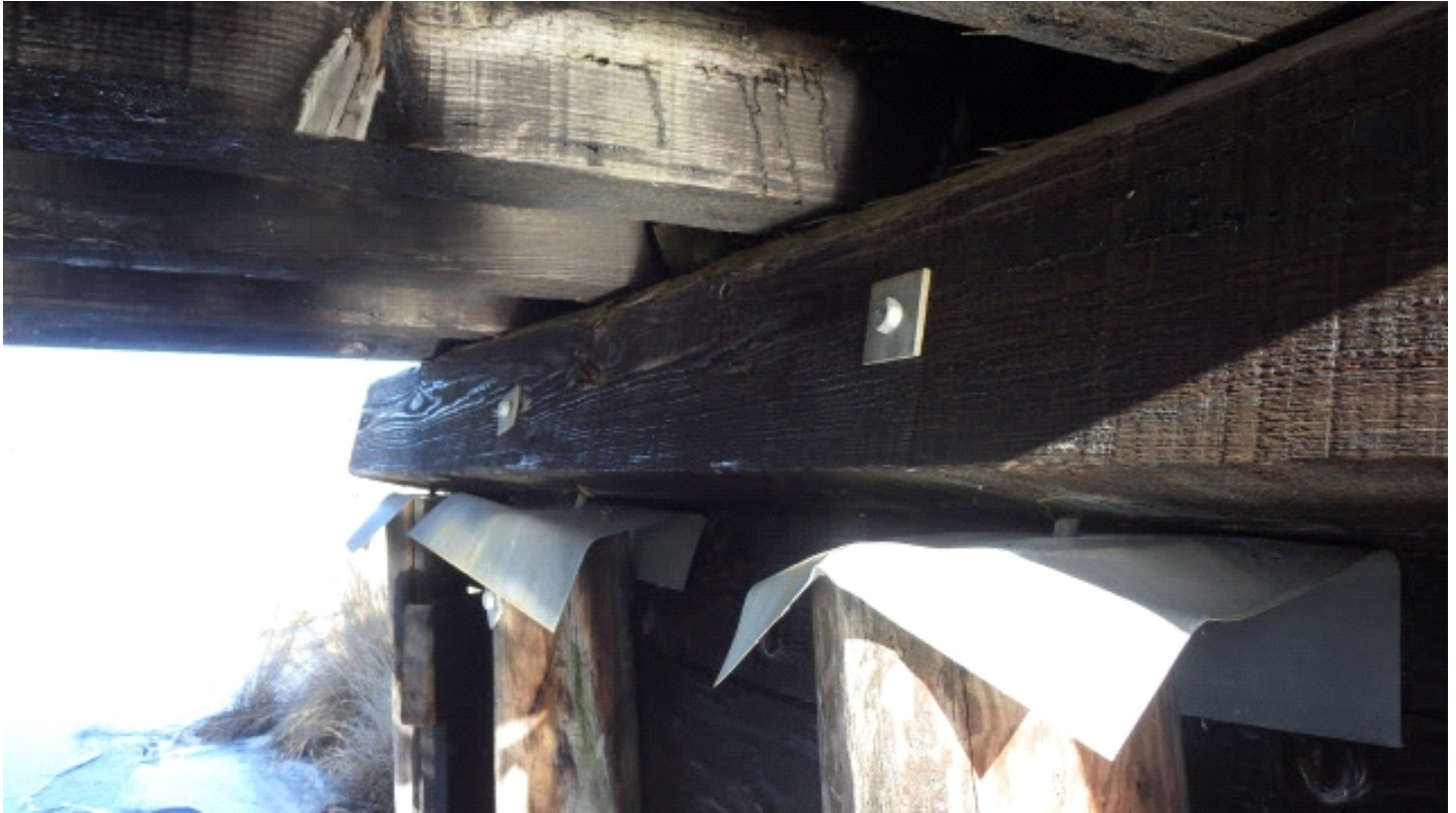
South pile cap, no bearing on piles
