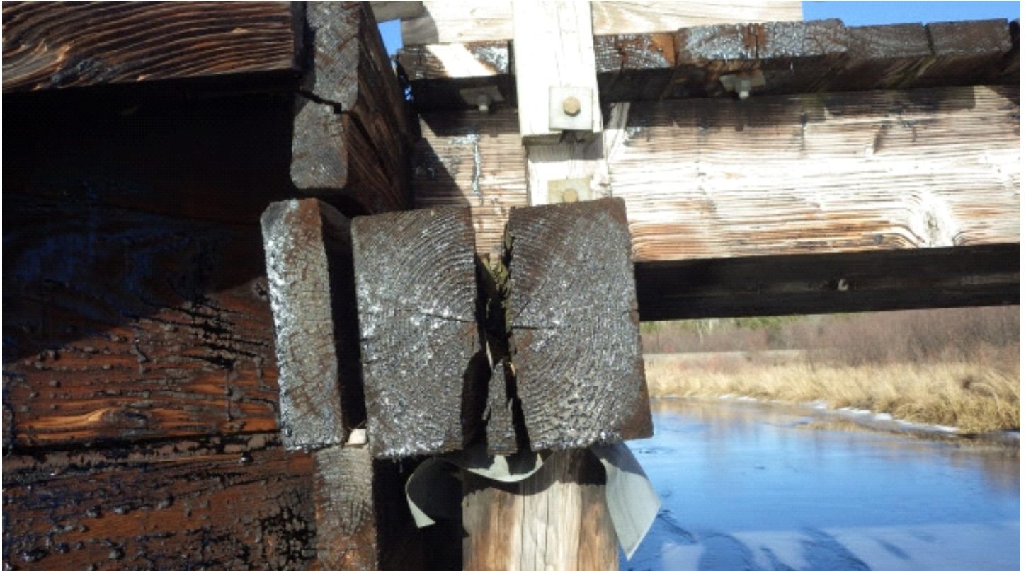
West end of north pile cap severely split through and moderate tilt backwards
