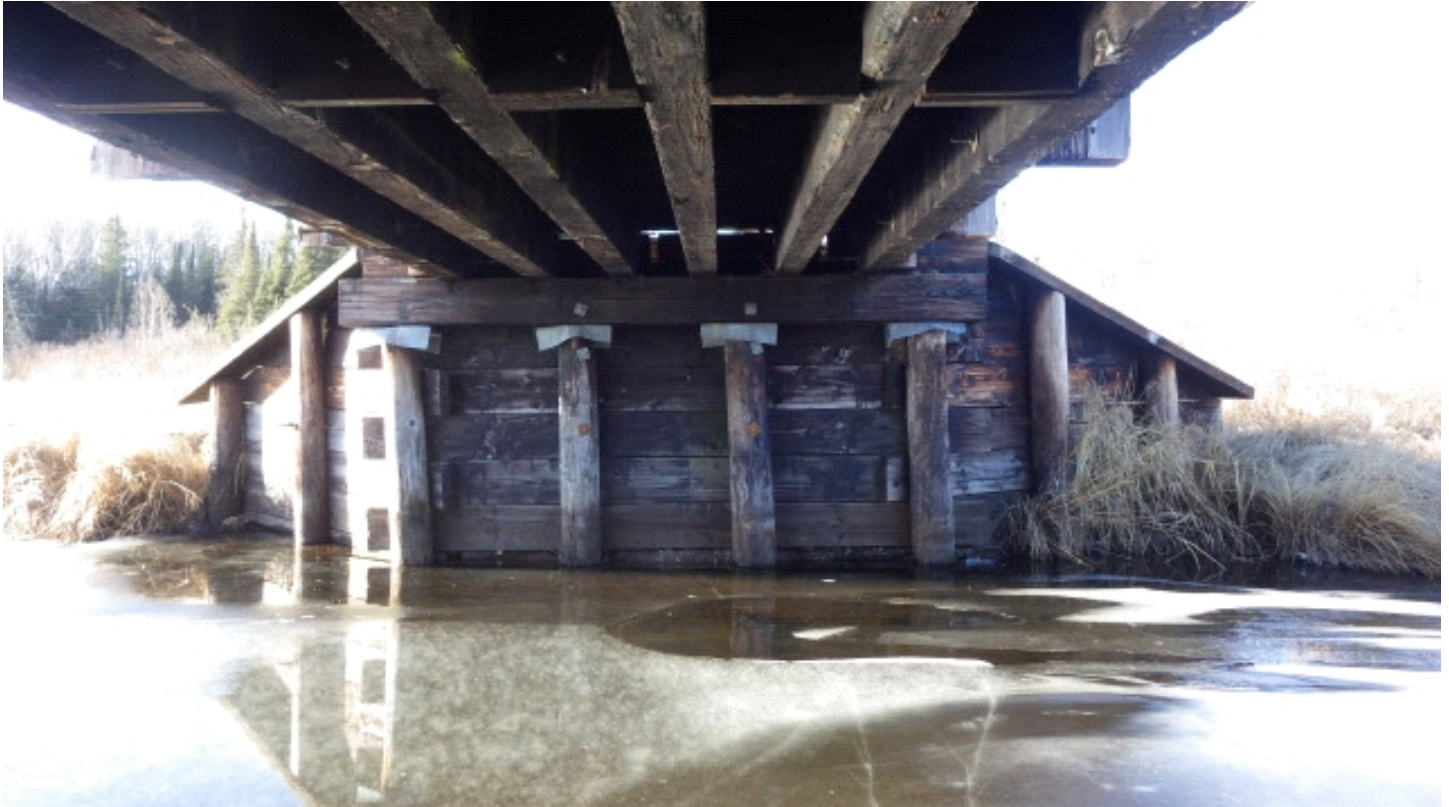
North abutment elevation (undermined backing boards)
