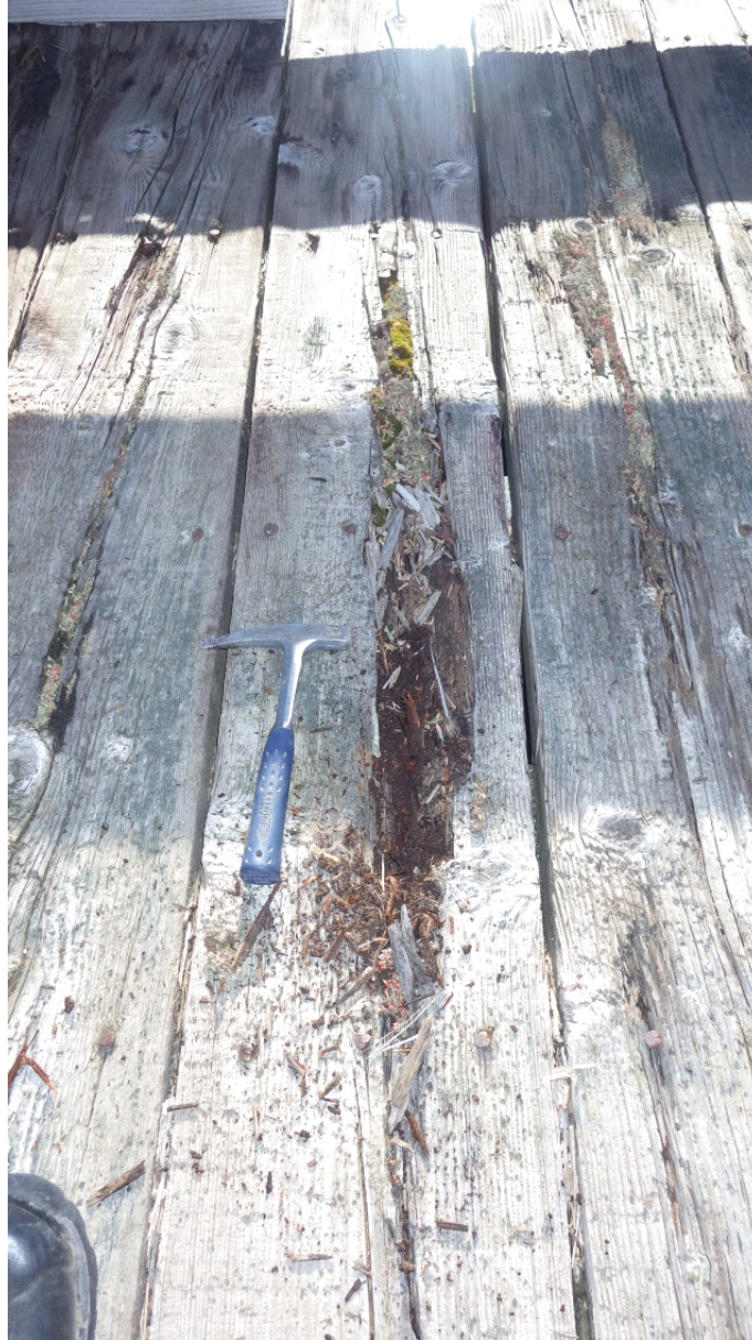
Entire deck rotten
