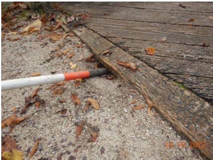
Minor sinkhole at the north approach.
