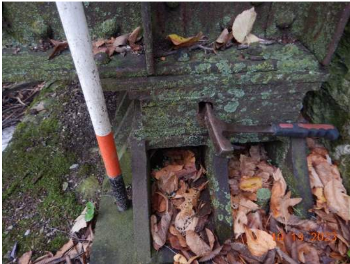
Hole in filler plates at SW bearing.
