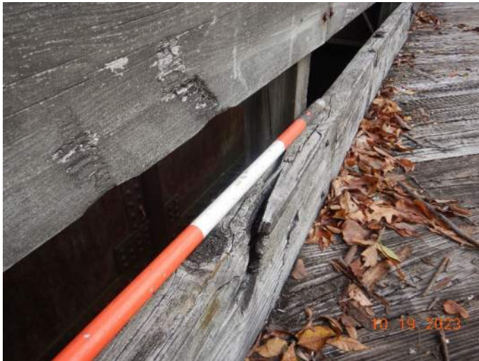
Split toe rail in the NE quadrant.
