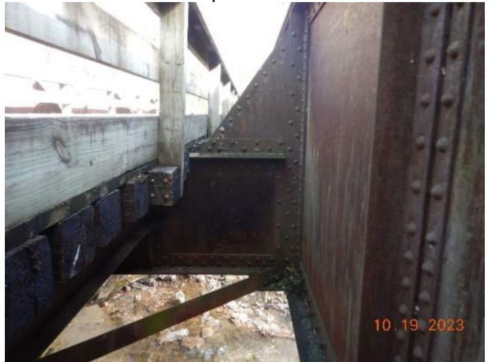
Typical minor surface corrosion of all steel members. Overview of floor beam through truss connection.
