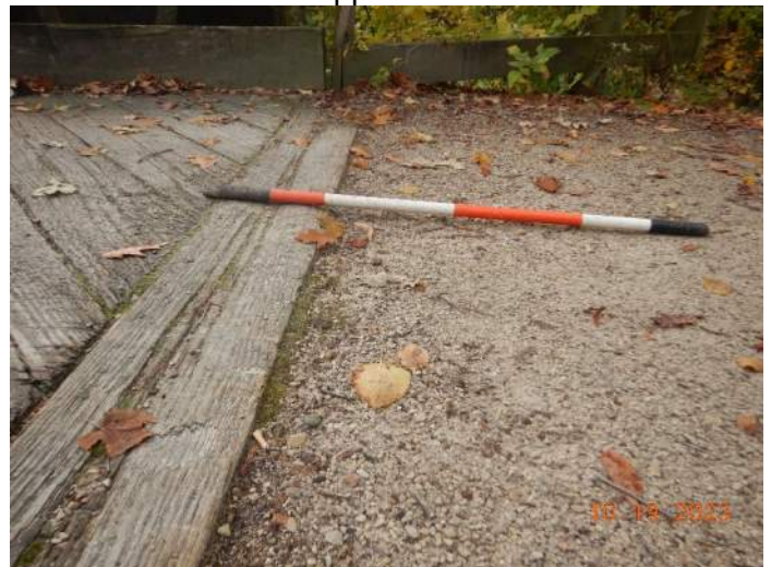
Typical settlement of gravel approaches (south shown).
