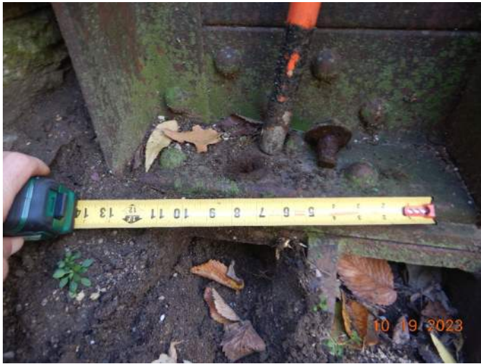
Broken keeper rod at the NW bearing
