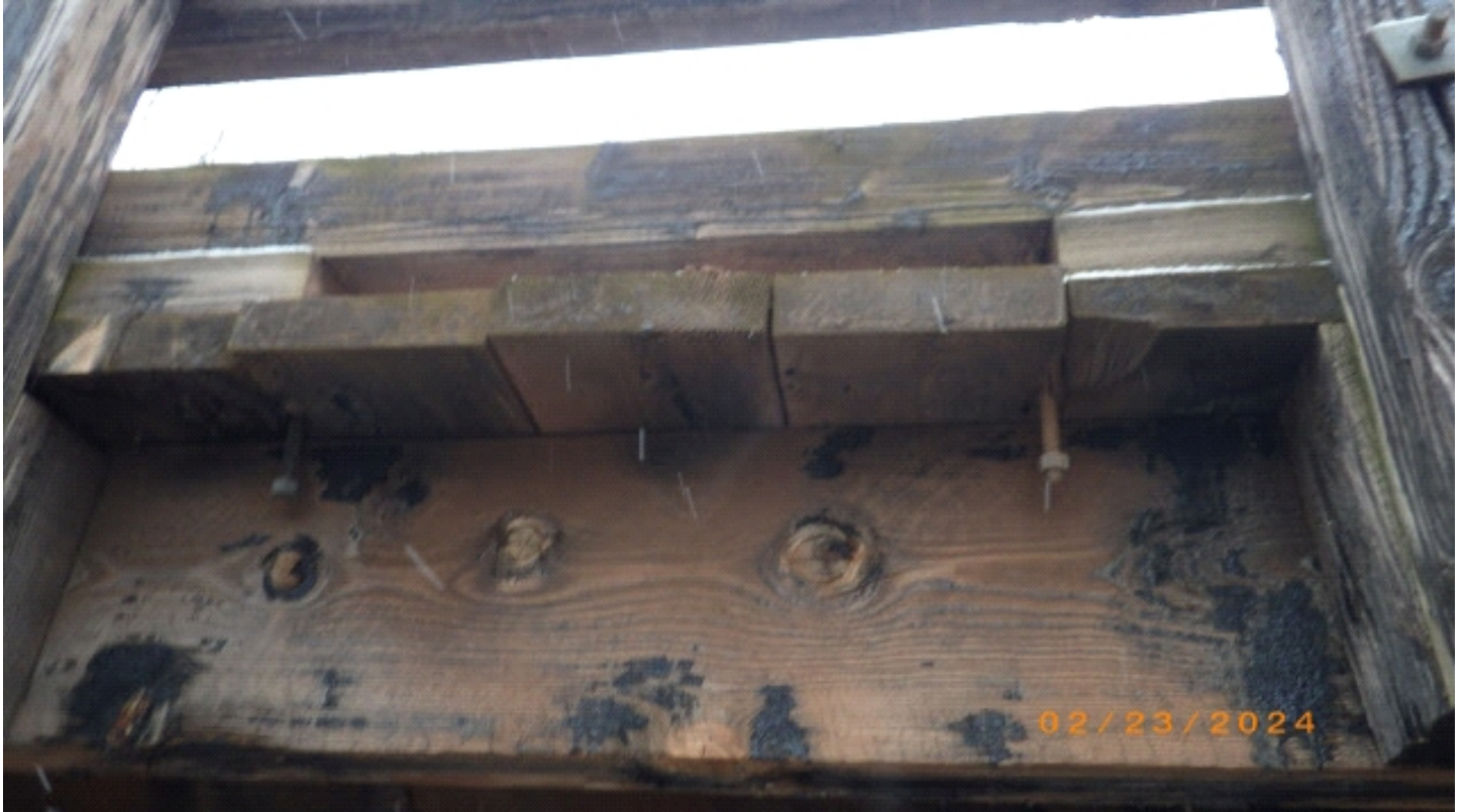
Curb bolts loose.
