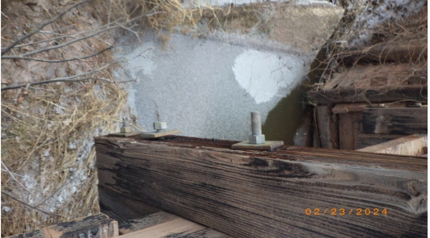
Loose rail hardware
