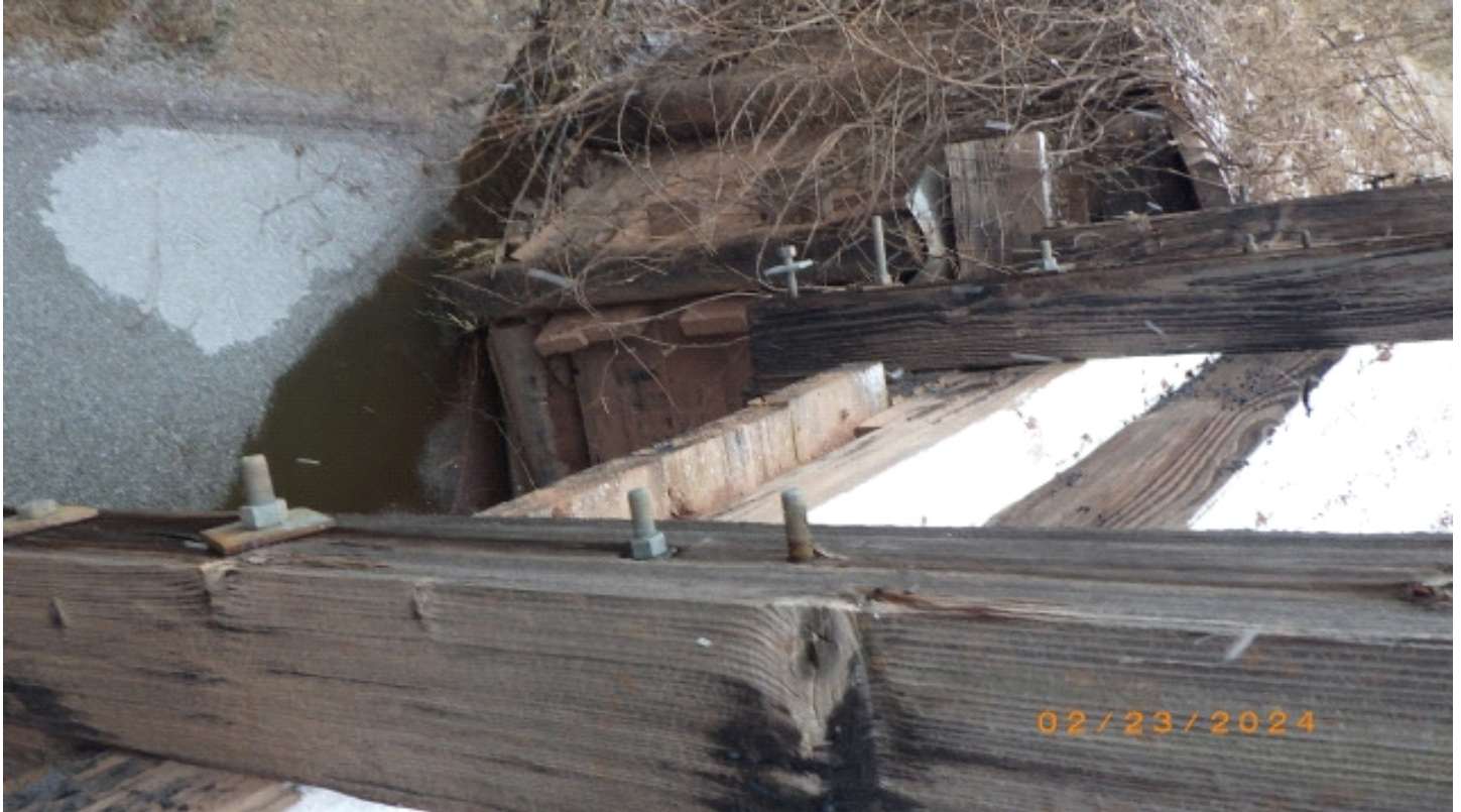
Missing rail hardware
