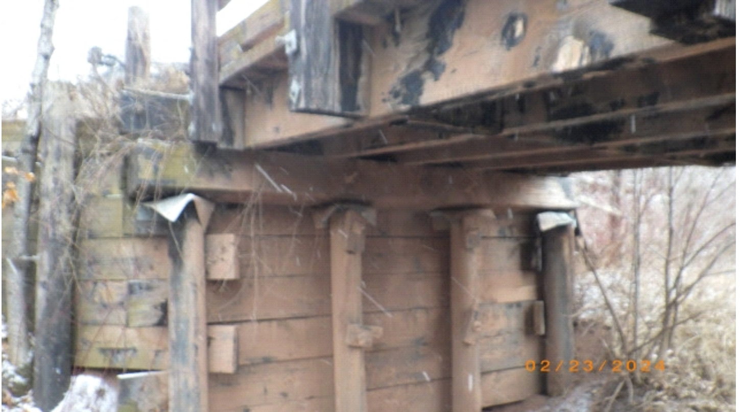
East Pile cap not touching 90% of the length.
