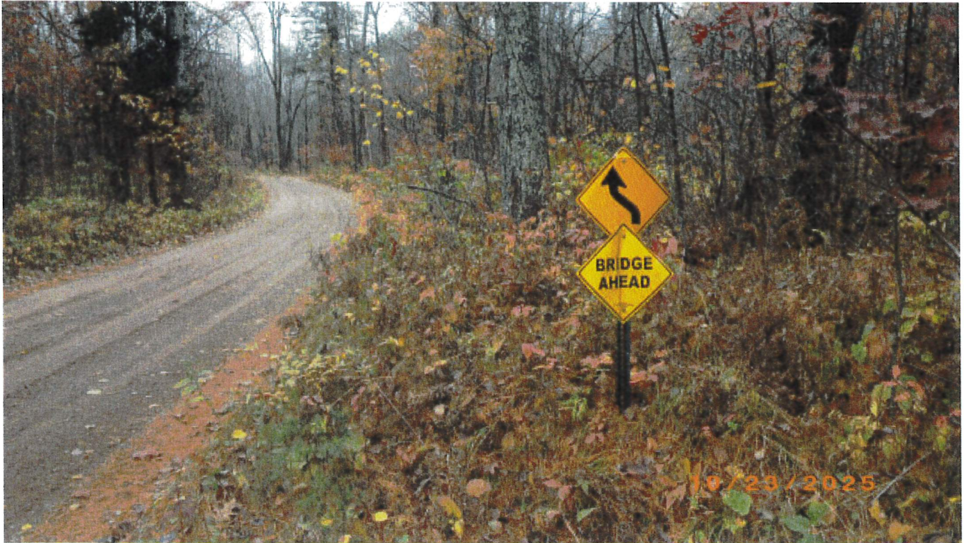
South bridge ahead sign, CS3 damage
