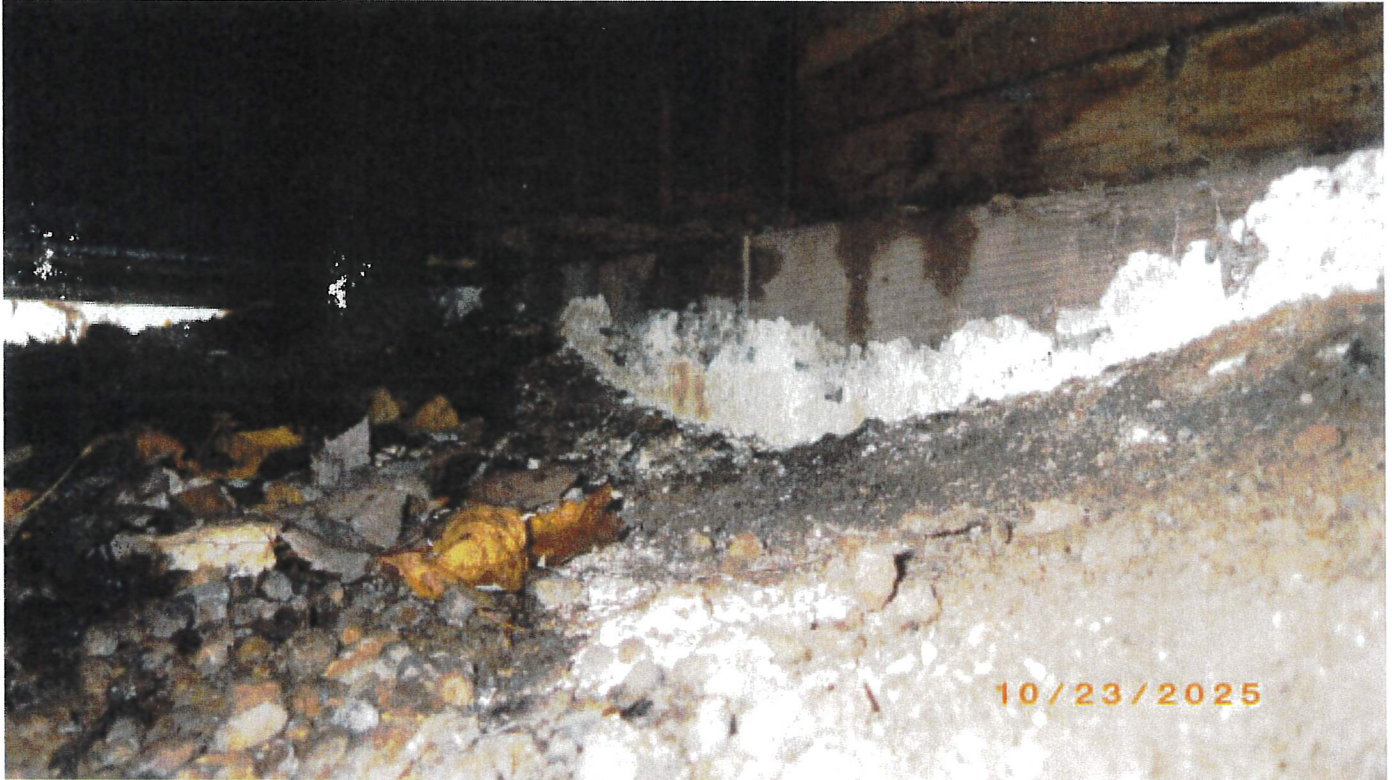
North sill white rot
