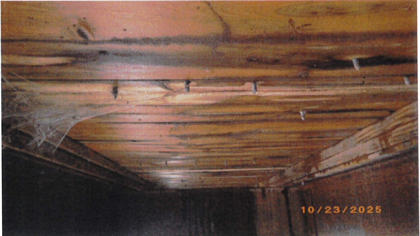
Line of cracked deck planks under west wheel path
