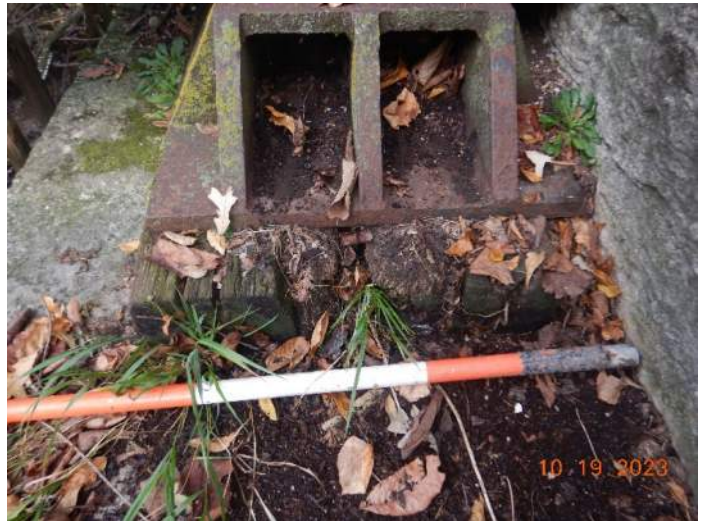
Rotten timber bearing pad under the NE bearing.
