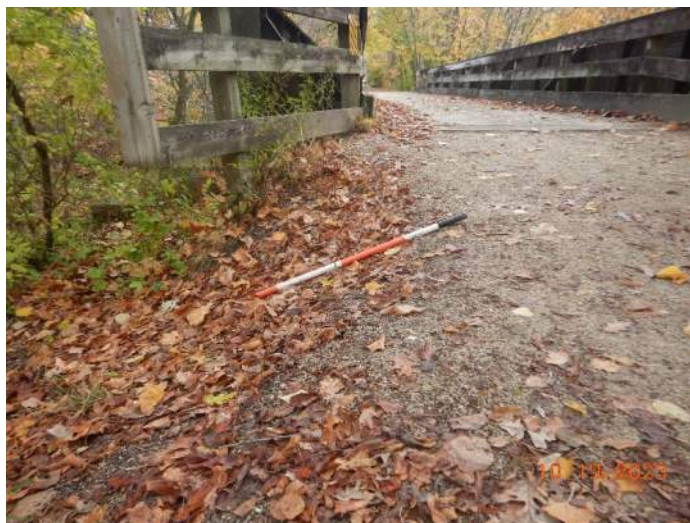
Erosion and settlement of shoulder and approach slope in SW quadrant.
