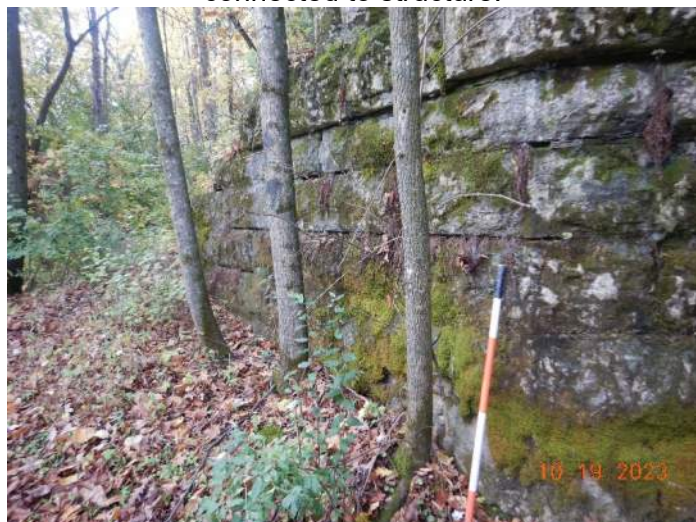
Typical tree growth along wingwalls (fascia similar).
