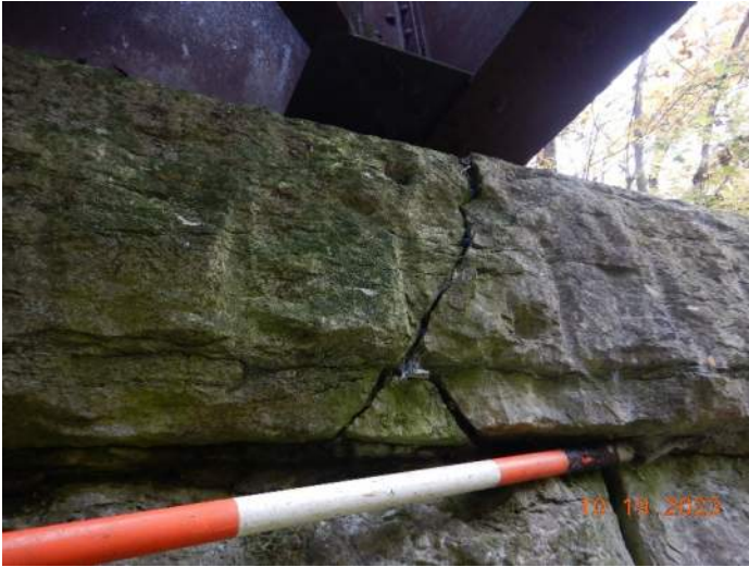
Wide crack in abutment stone cap at north abutment east end.
