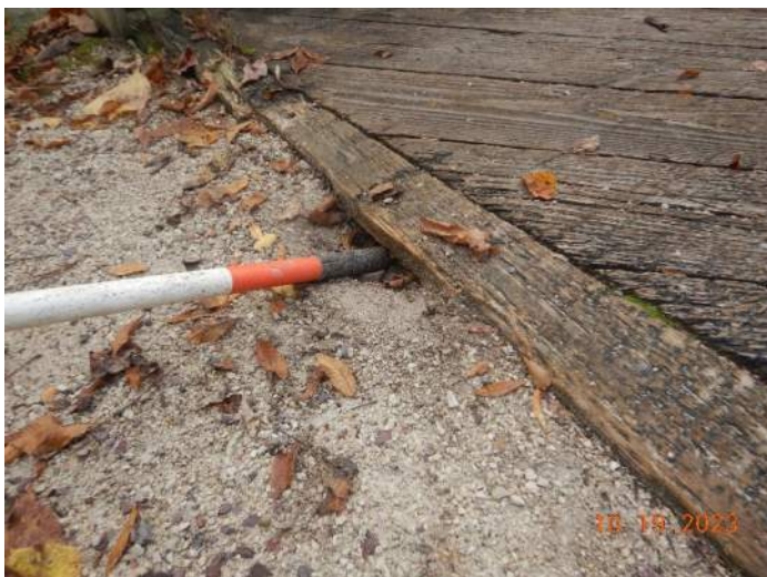
Minor sinkhole at the north approach.
