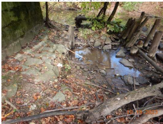
Minor to moderate scour in front of south abutment.
