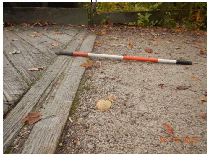
Typical settlement of gravel approaches (south shown).
