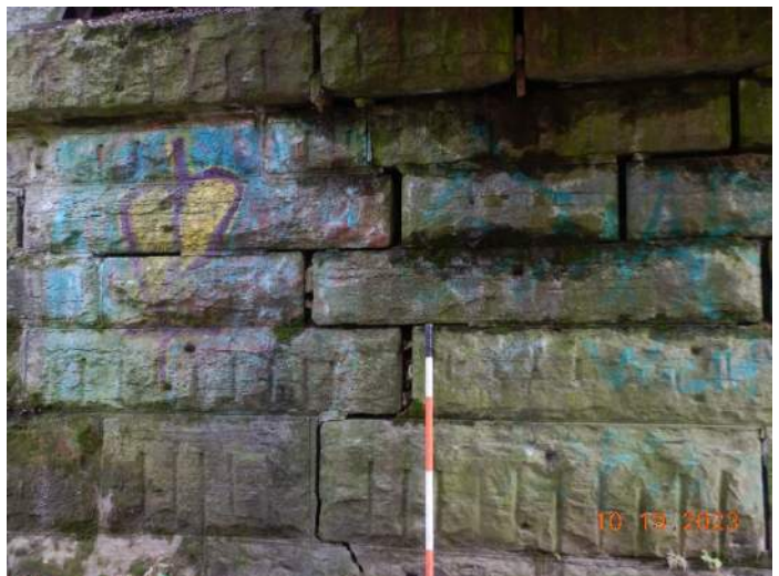
Typical missing mortar in joints at north abutment (south abutment similar).
