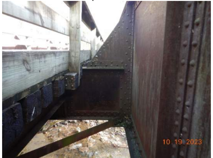
Typical minor surface corrosion of all steel members. Overview of floor beam through truss connection.
