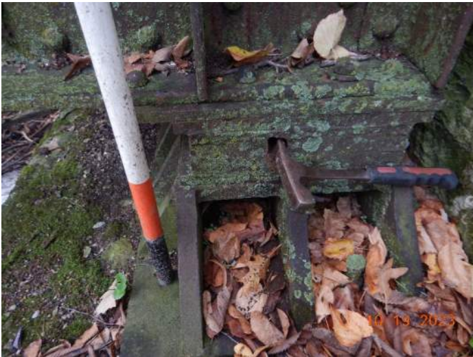
Hole in filler plates at SW bearing.
