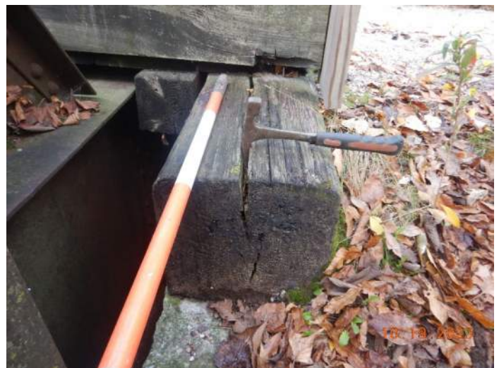
Typical timber cap split and rotten (NE quadrant shown).
