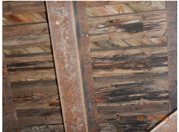
Typical deterioration of timber railroad ties.
