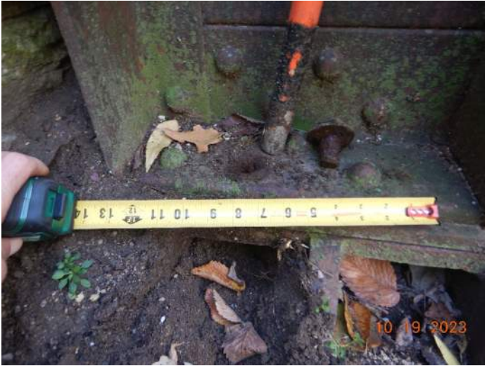
Broken keeper rod at the NW bearing
