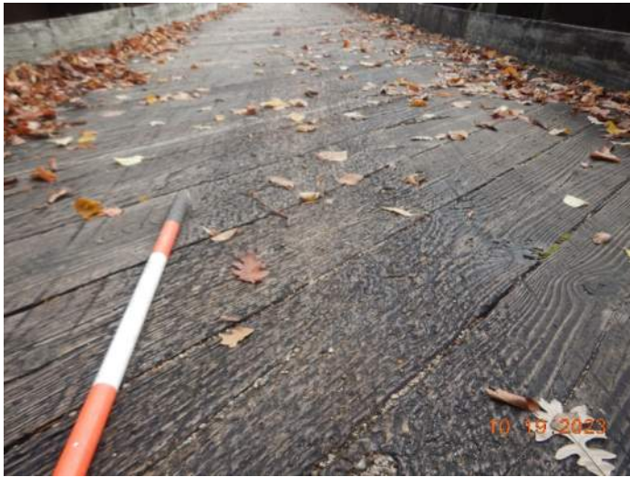
Moderate to heavy wear of deck boards down centerline.
