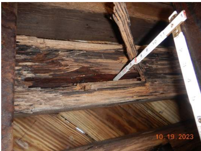
Typical deterioration, severe rot, and section loss of timber railroad ties.
