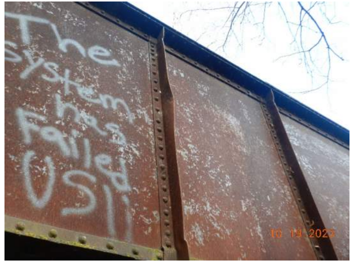
Bent outside stiffener east through girder south end.
