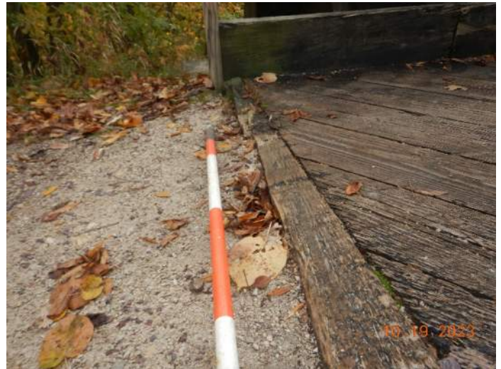
Split and portion missing timber header at north approach.
