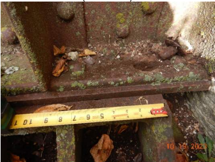
Broken keeper rod at the NE bearing.
