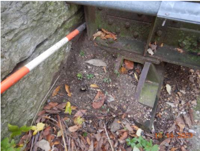
Typical debris and sediment buildup around bearing (NW shown).
