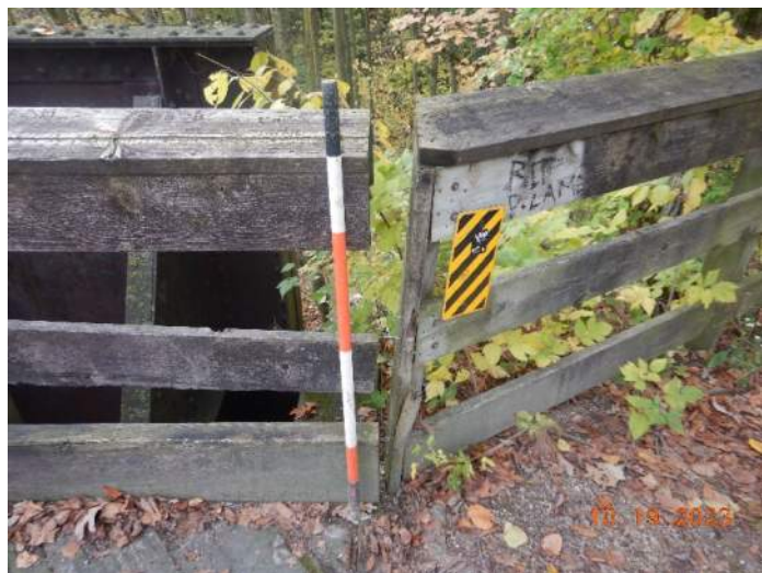
Typical approach rail in south approach not connected to structure.
