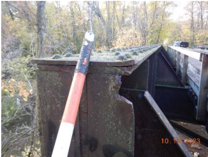
Minor damage to through girder NE quadrant.
