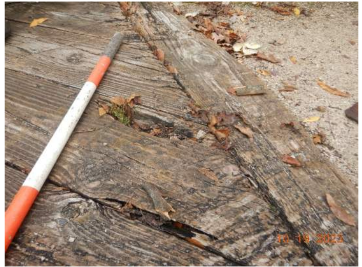
Rotten timber deck boards with minor section loss at north end.
