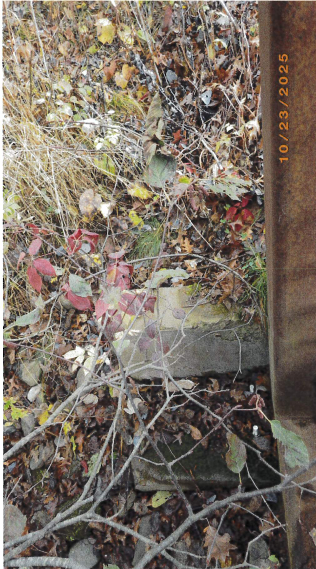
CS3 spalling on north end of east sill.
