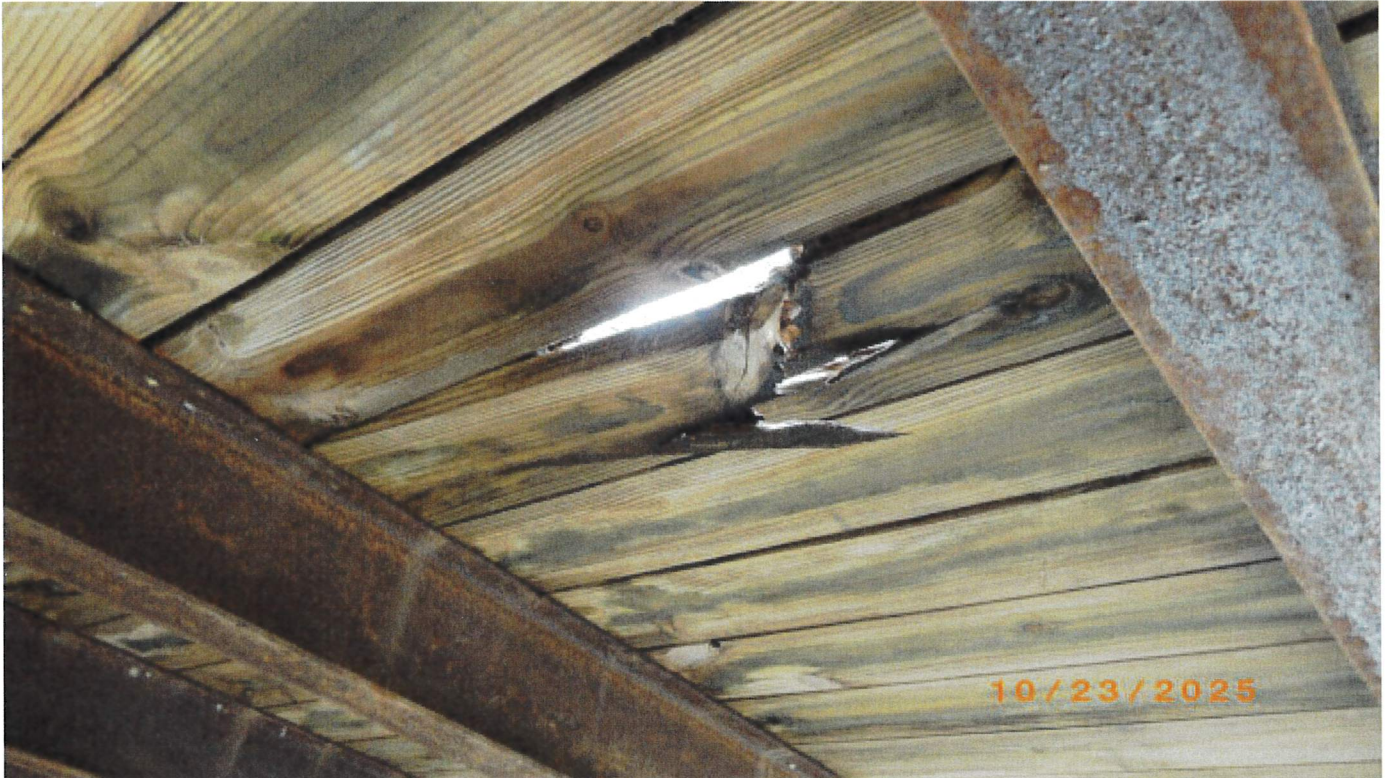
Hole through decking from below.
