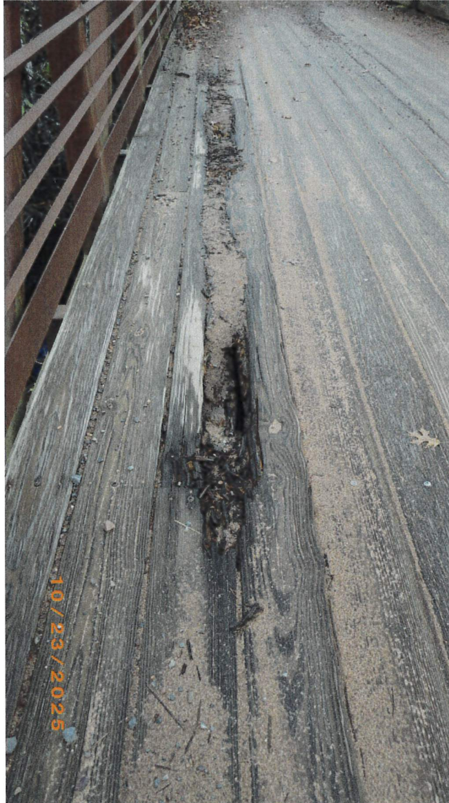
Hole through wear planks and decking in NE corner.
