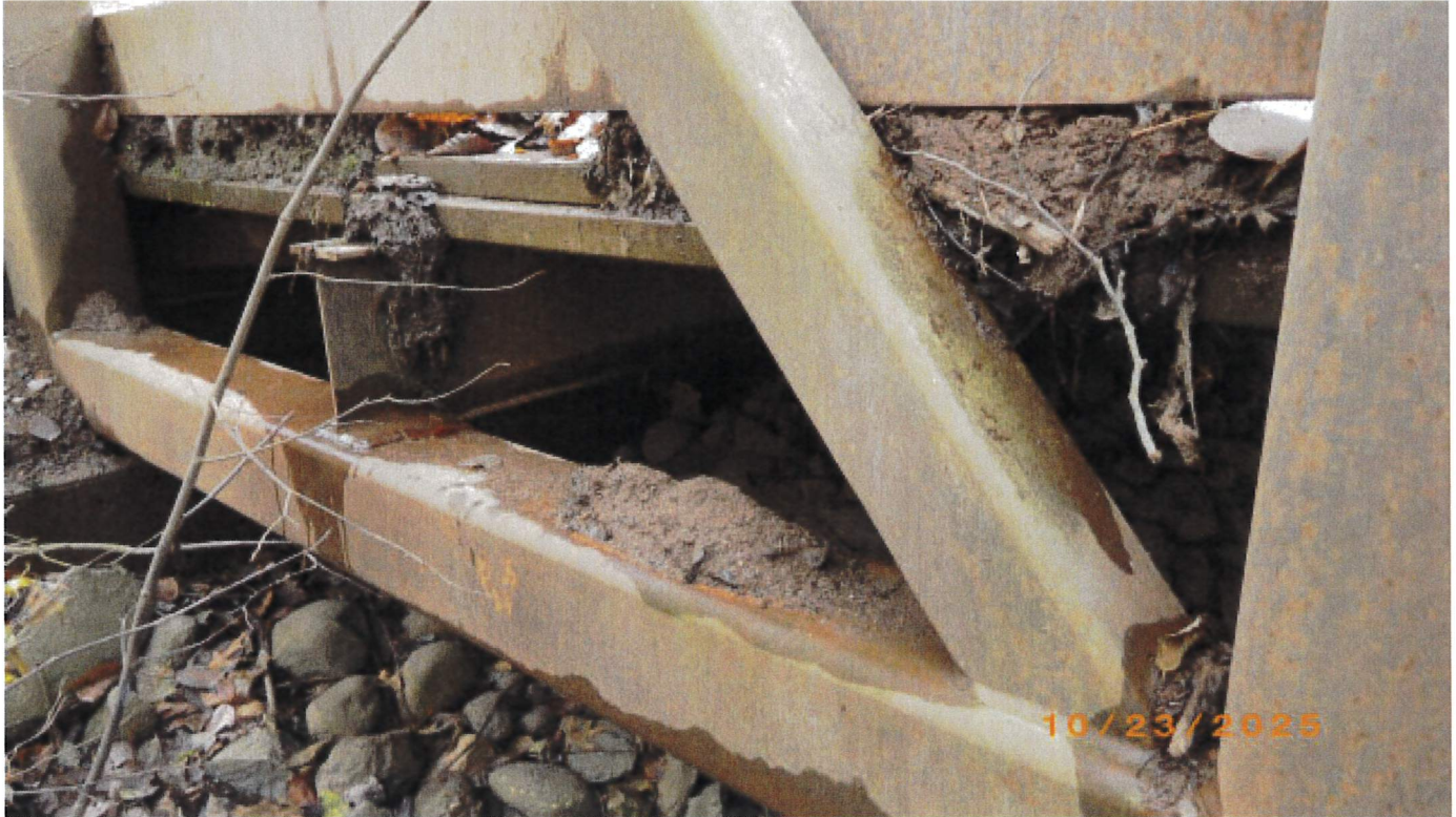
Sand on low chord ends
