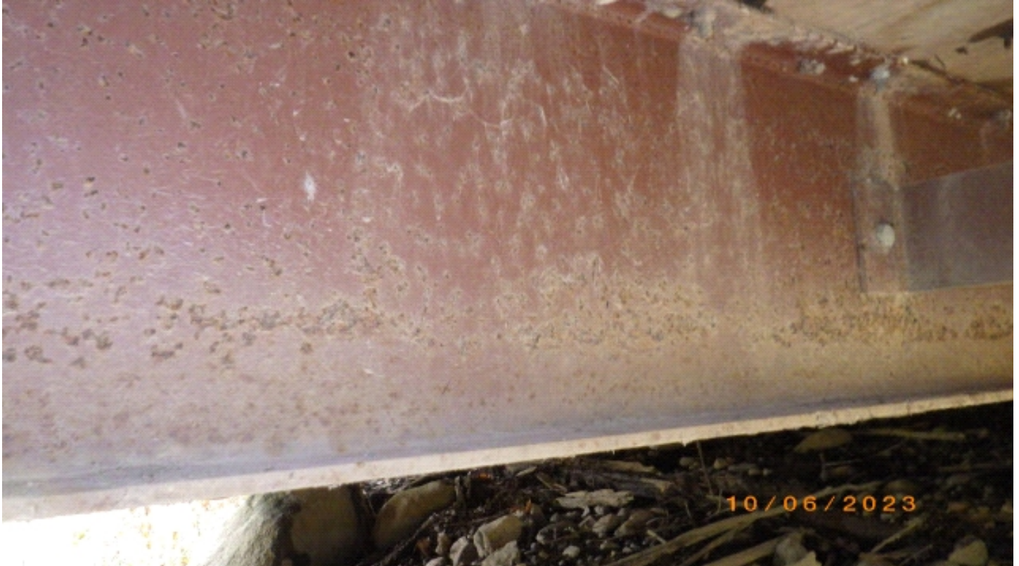
CS2 corrosion, typ.
