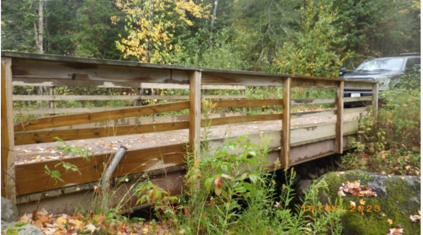
Looking West, damaged railing.
