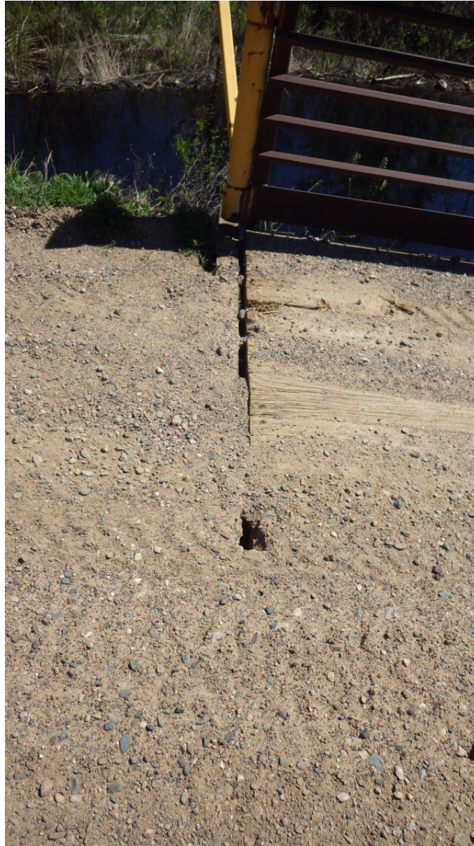
Gap between backwall and deck, north end
