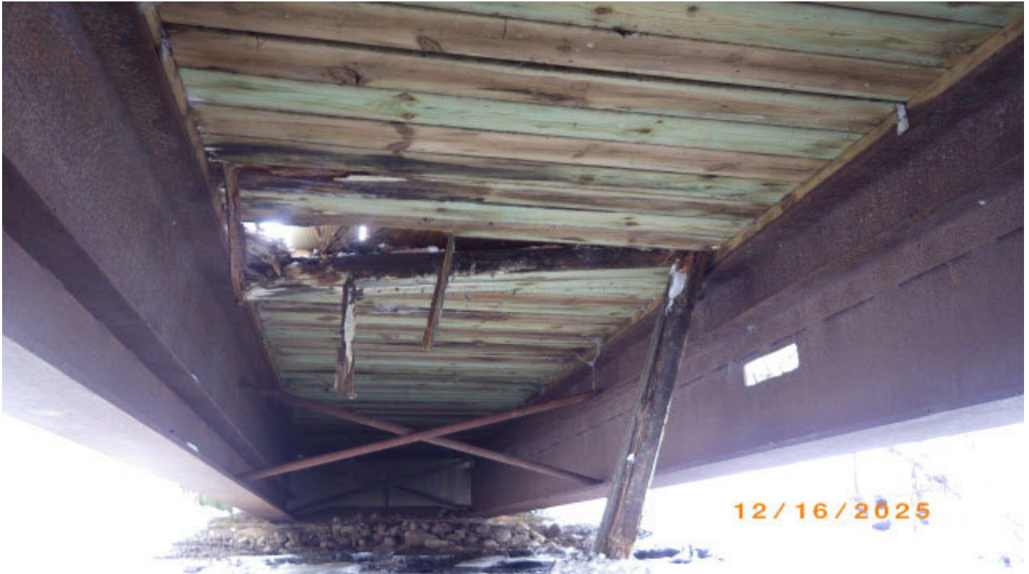
Typical deck / superstructure underside with large deck failure in center
