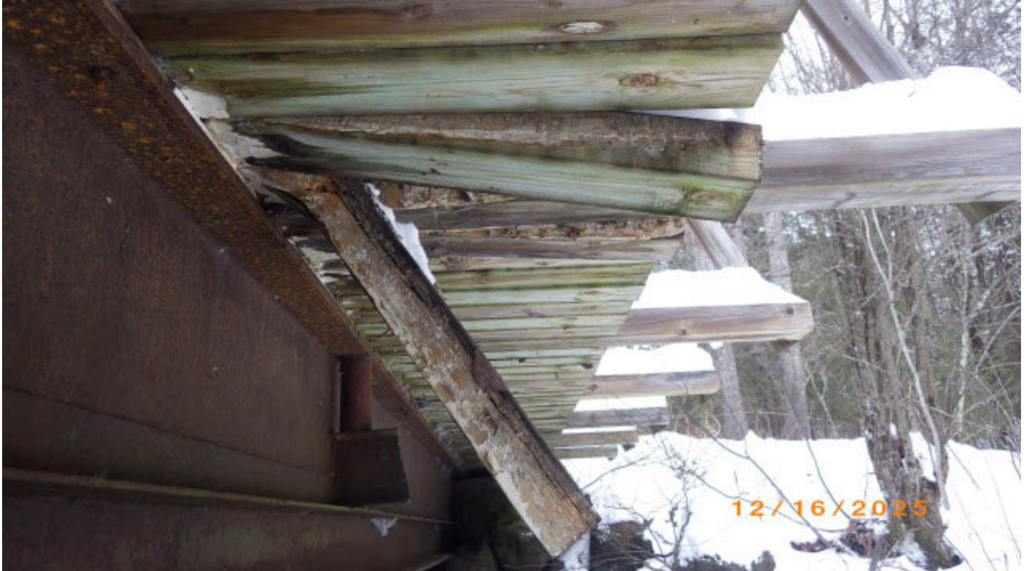
CS4 deck overhang failures
