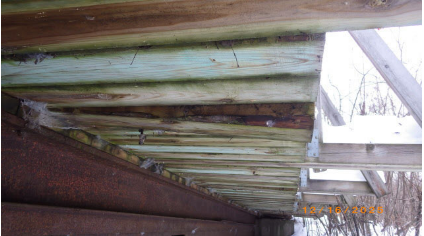
Downstream girder / deck overhang partial failures
