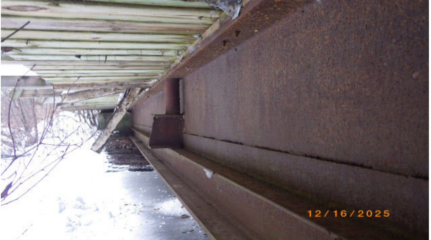
Upstream girder fascia / failed deck overhang planks
