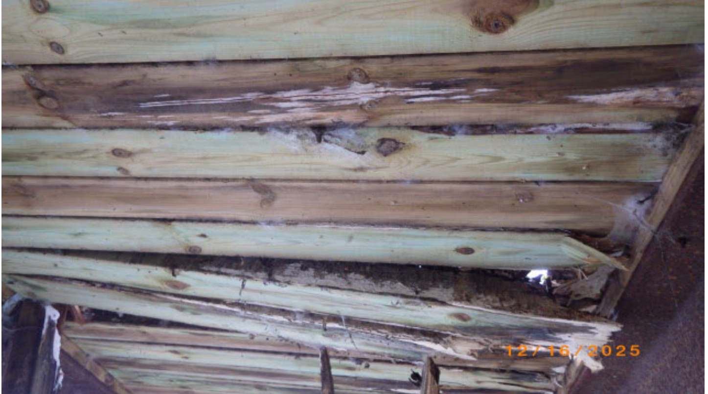
CS4 deck decay and failures
