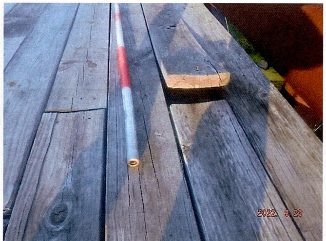
West Span Warped Deck Plank
