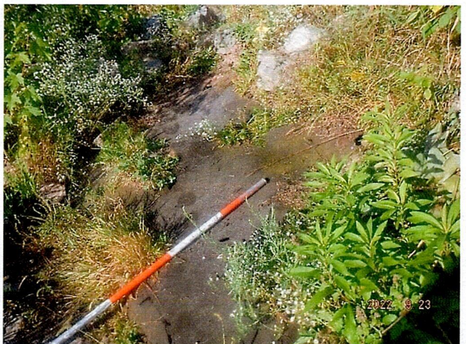
West Abutment Bare Slope. Fabric Exposed
