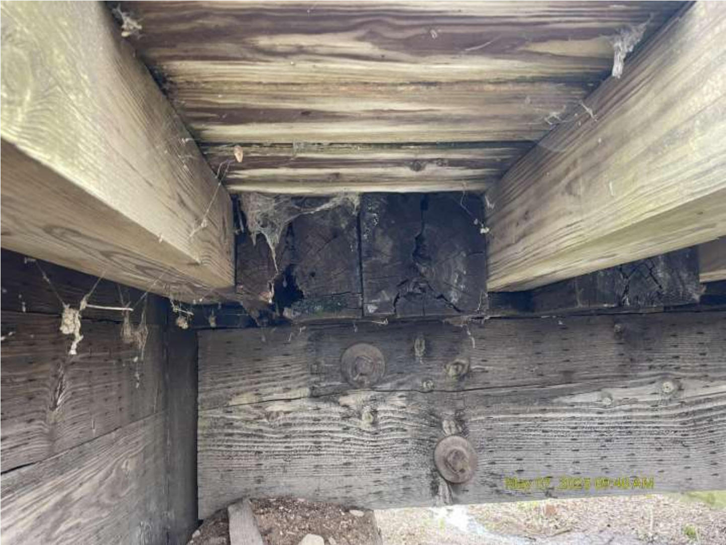
West RR ties rotted
