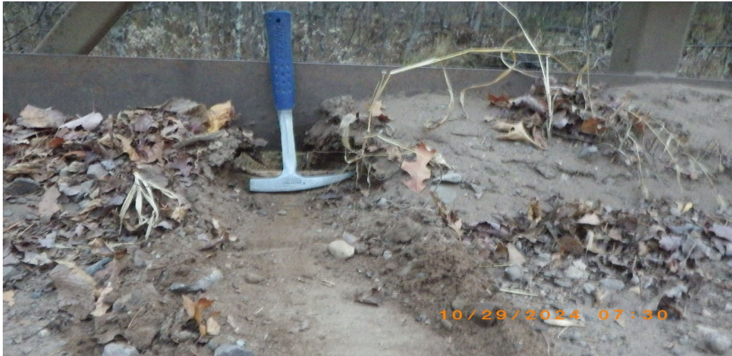
Excessive sand on deck
