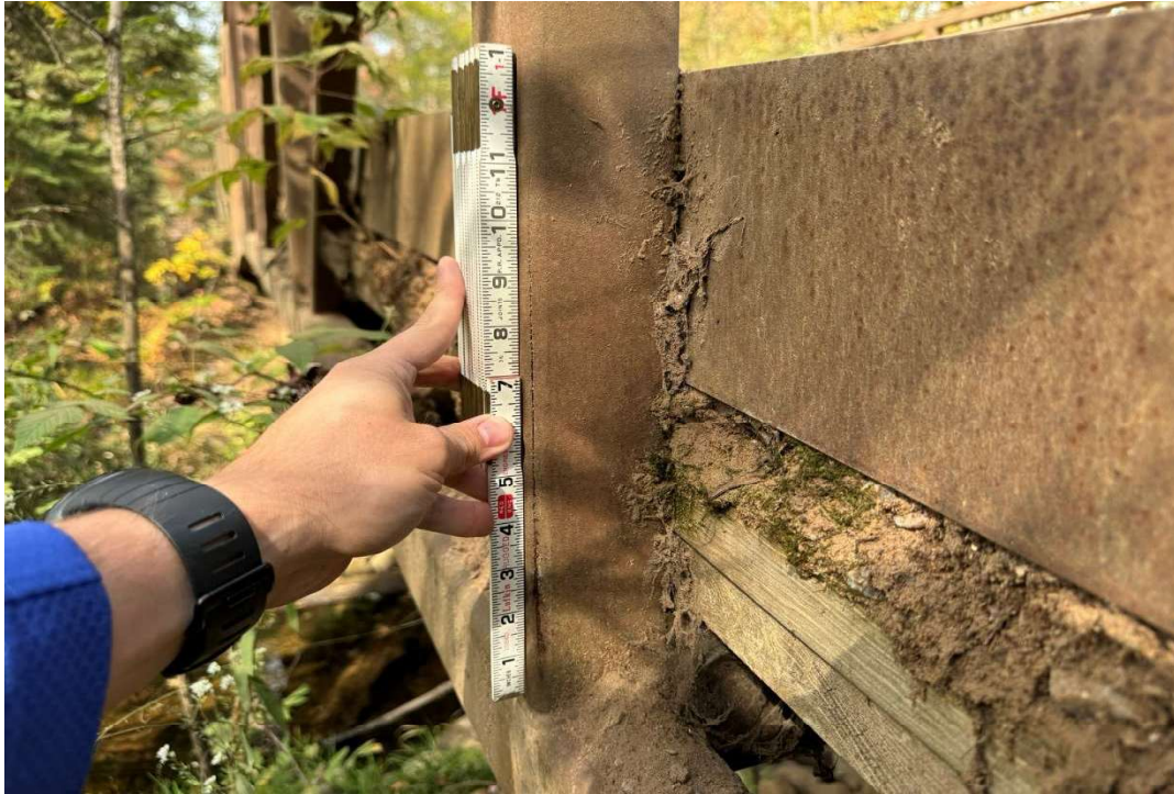
Closeup of L1 crack
