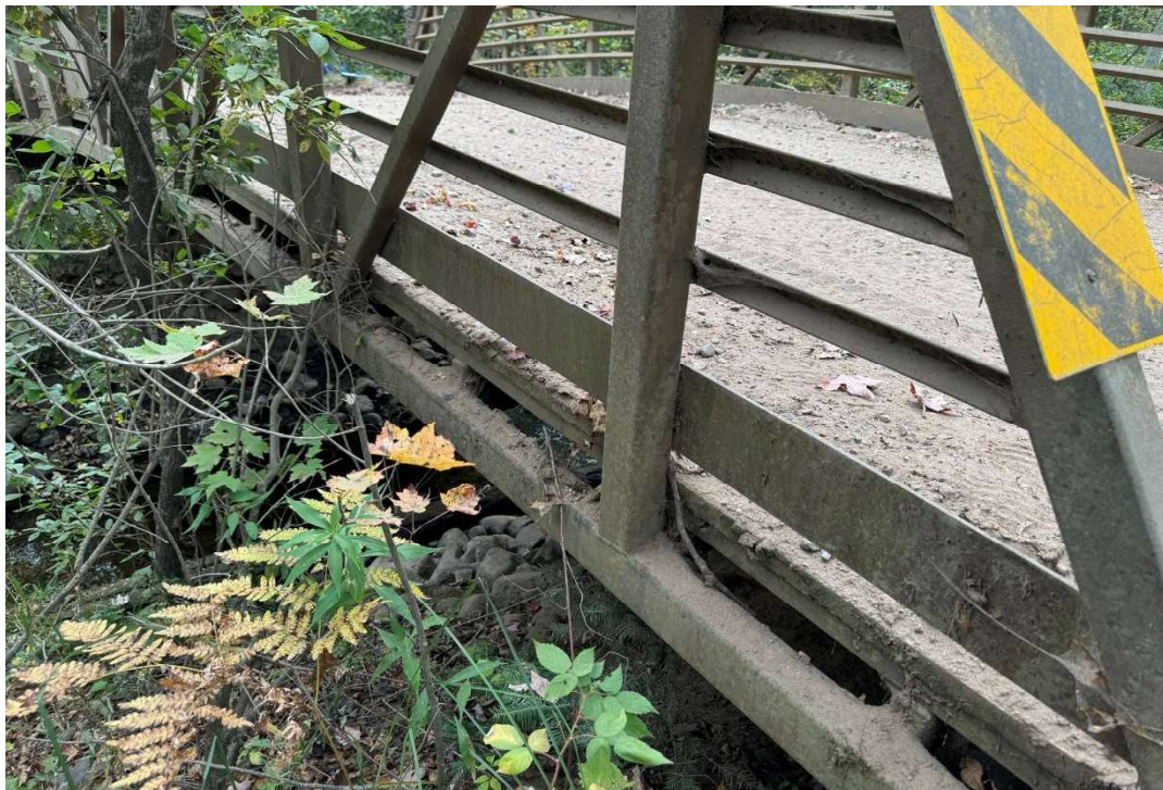
Toward R6 crack from NE quad
