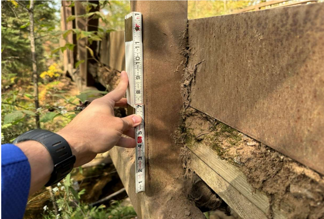
Closeup of L1 crack
