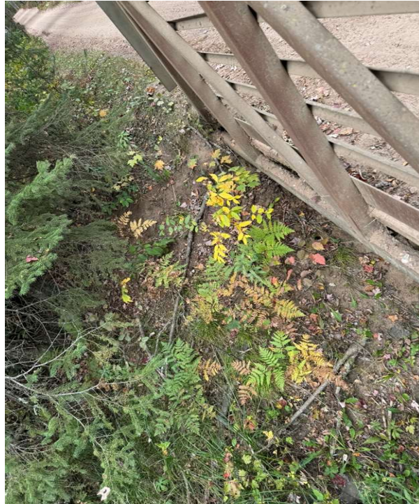
Toward crack at L6
