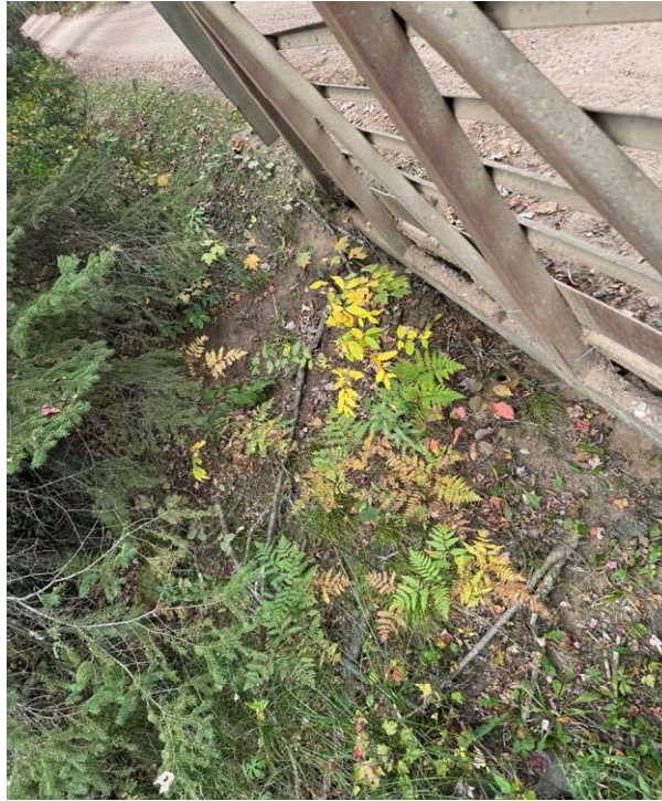
Toward crack at L6
