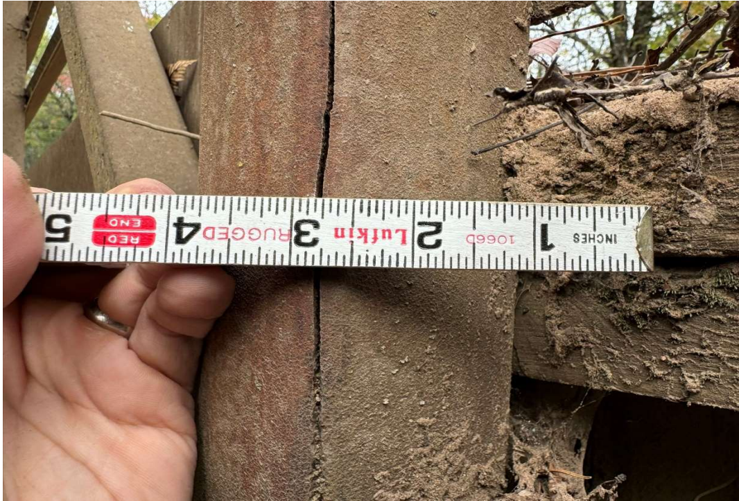
Another view of crack width at L6
