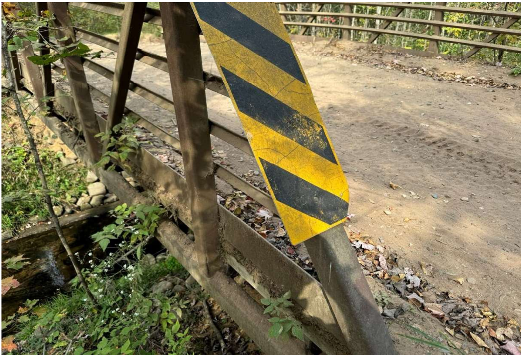
Toward crack at L1 panel point (Left truss looking north (upstream truss), 1st panel pt)
