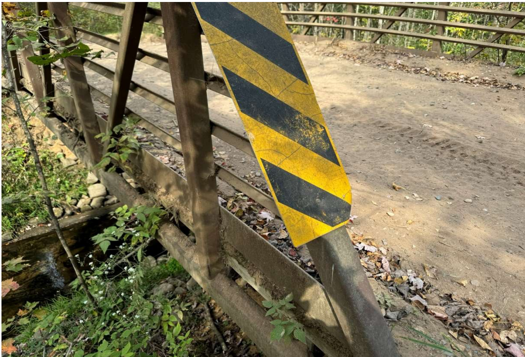
Toward crack at L1 panel point (Left truss looking north (upstream truss), 1st panel pt)
