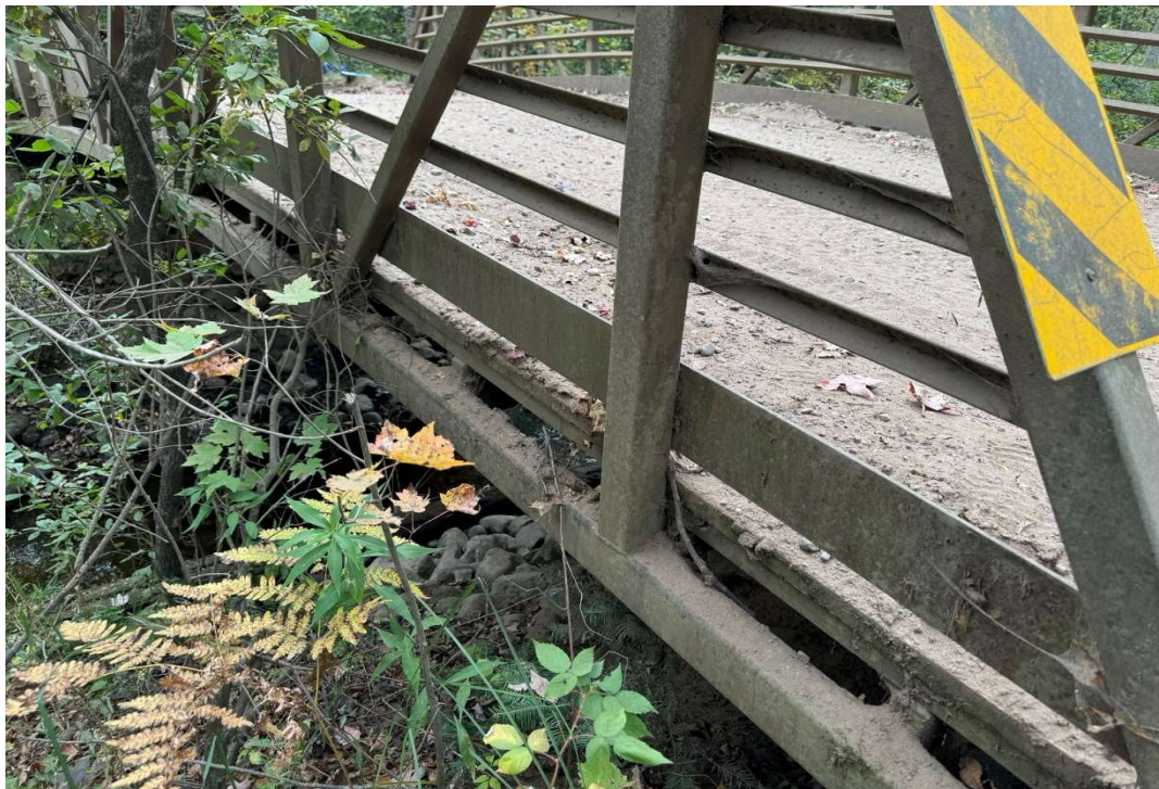
Toward R6 crack from NE quad
