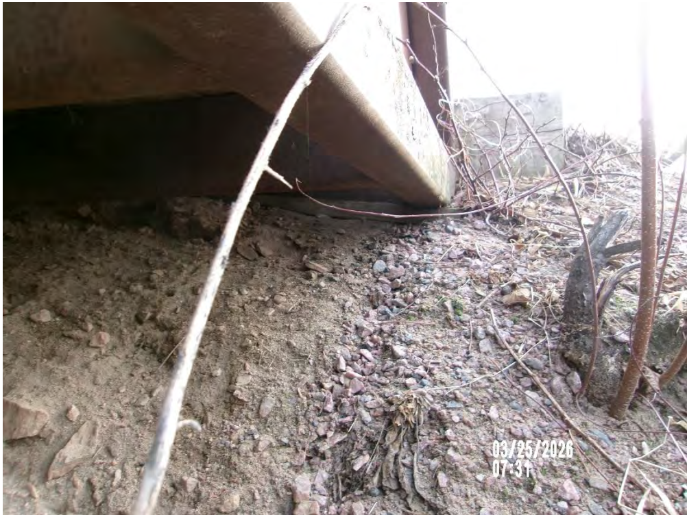
Figure 14: SE bearing board broken allowing sinking
