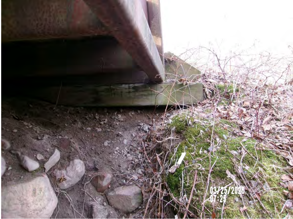
Figure 13: NW pier cap undermining
