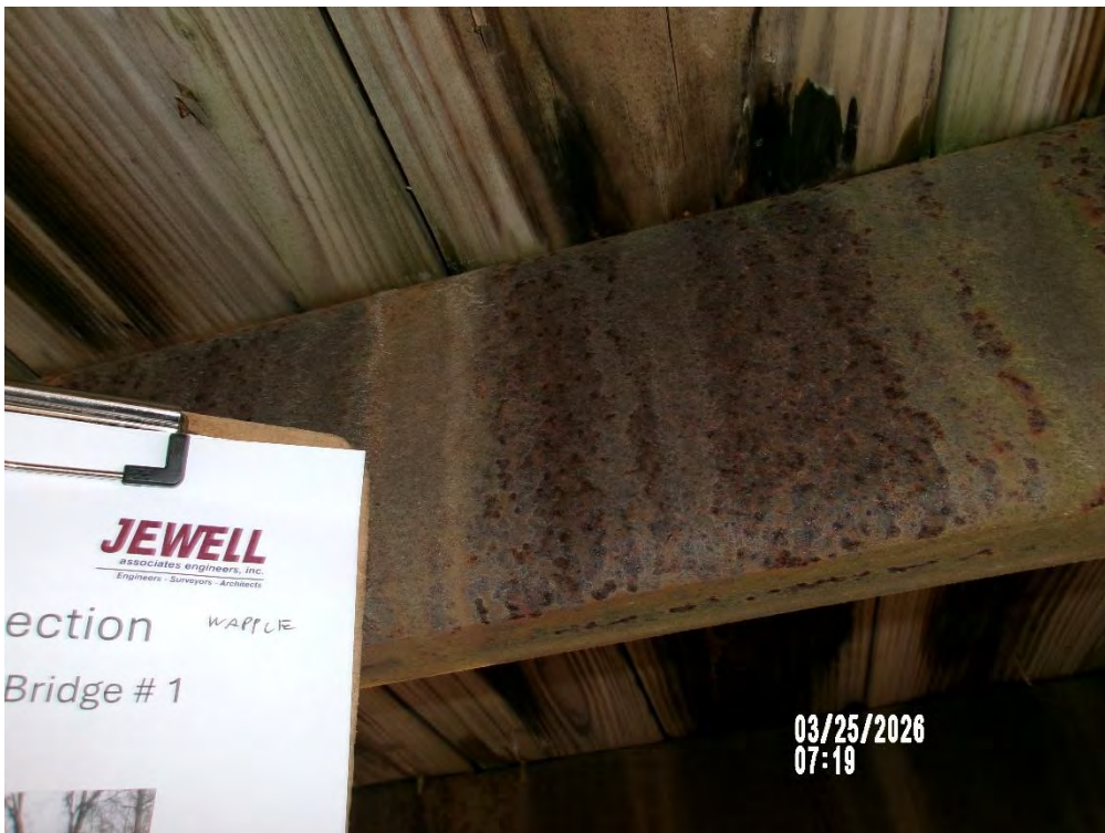
Figure 12: Worst case floor beam condition
