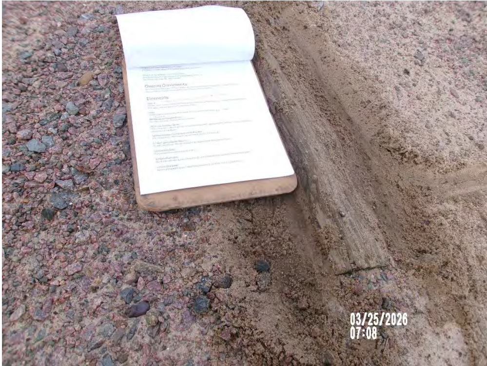
Figure 7: Settlement at East Abutment
