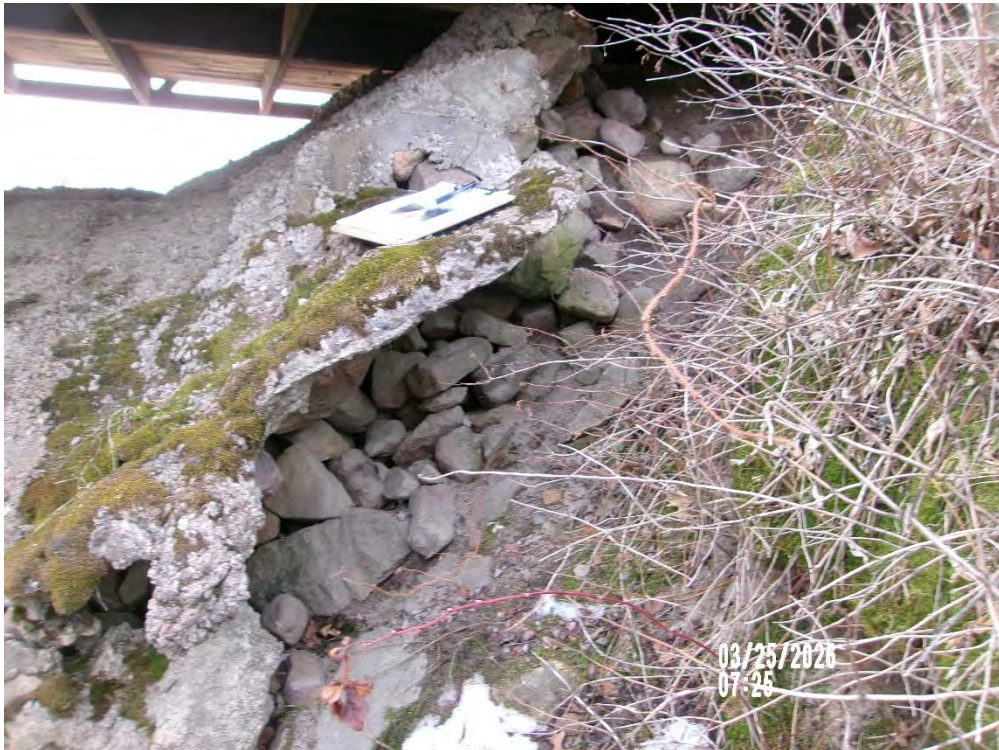
Figure 8: West slope protection undermining
