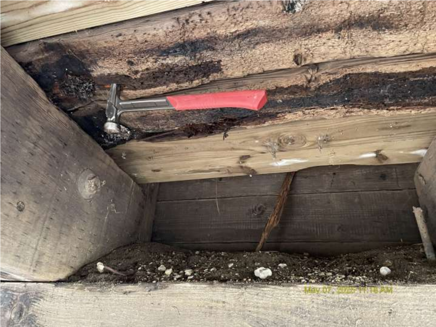
Rotted 8' x 8" RR tie at south abutment
