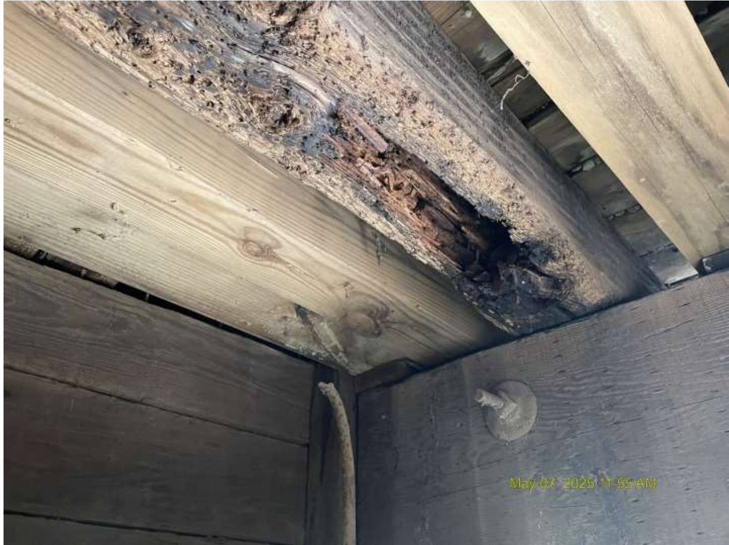
North end of bridge – rotted 8” x 8” RR ties
