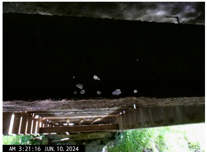
North I Beam Diaphragm with metal section loss & Holes
