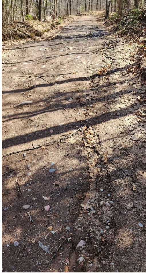
Hill 4: Water control structure in trail with washouts
