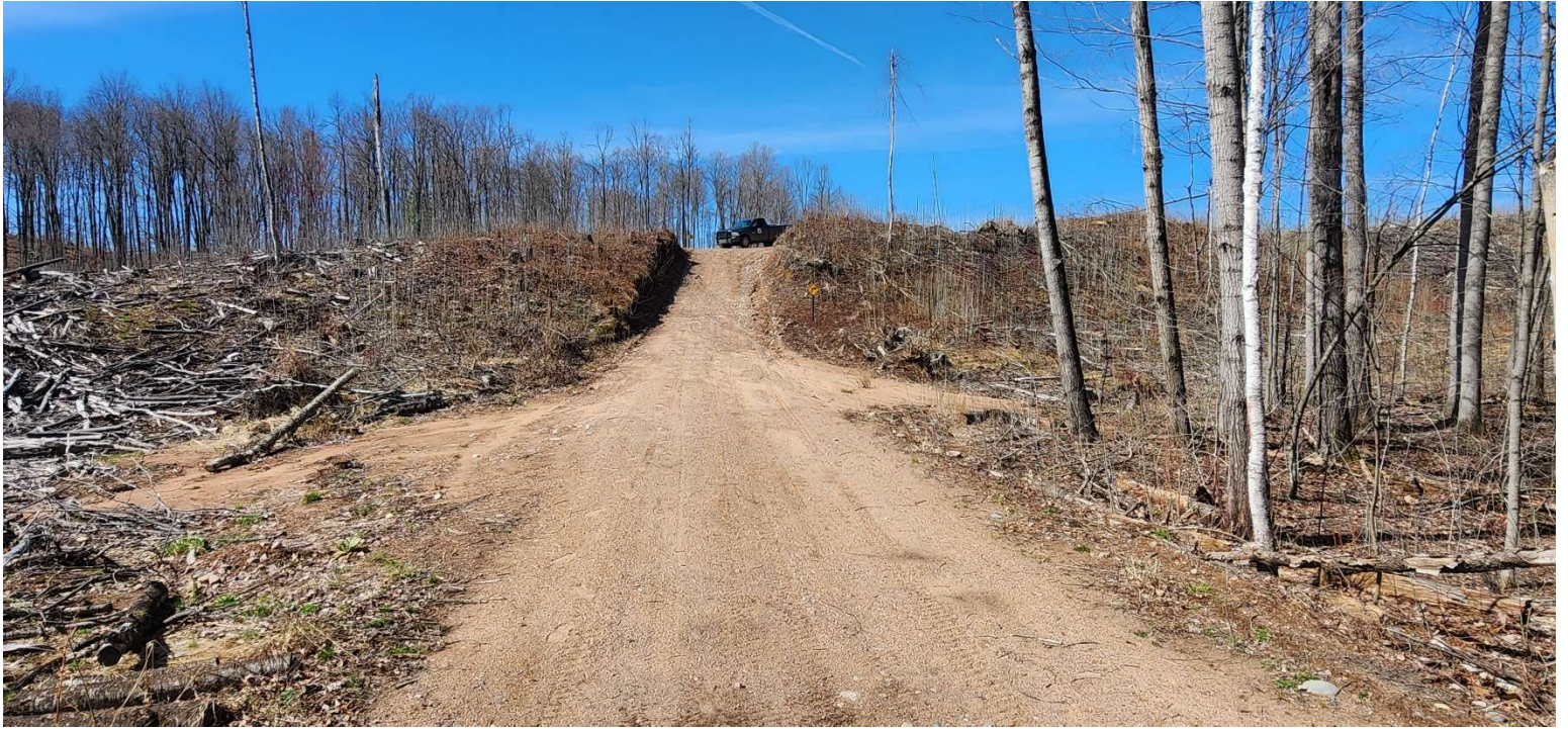
Hill 5: Washout erosion
