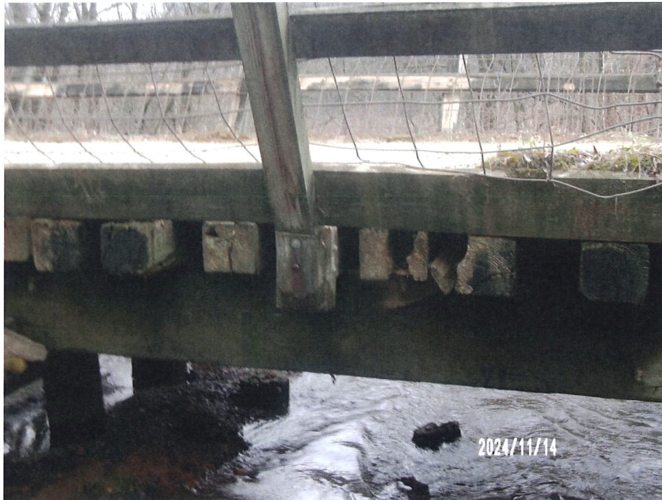
Figure 7: Timber Stringer Splitting
