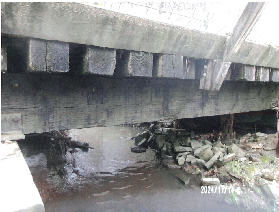
Figure 8: Narrow Split and Debris Damage on Girder
