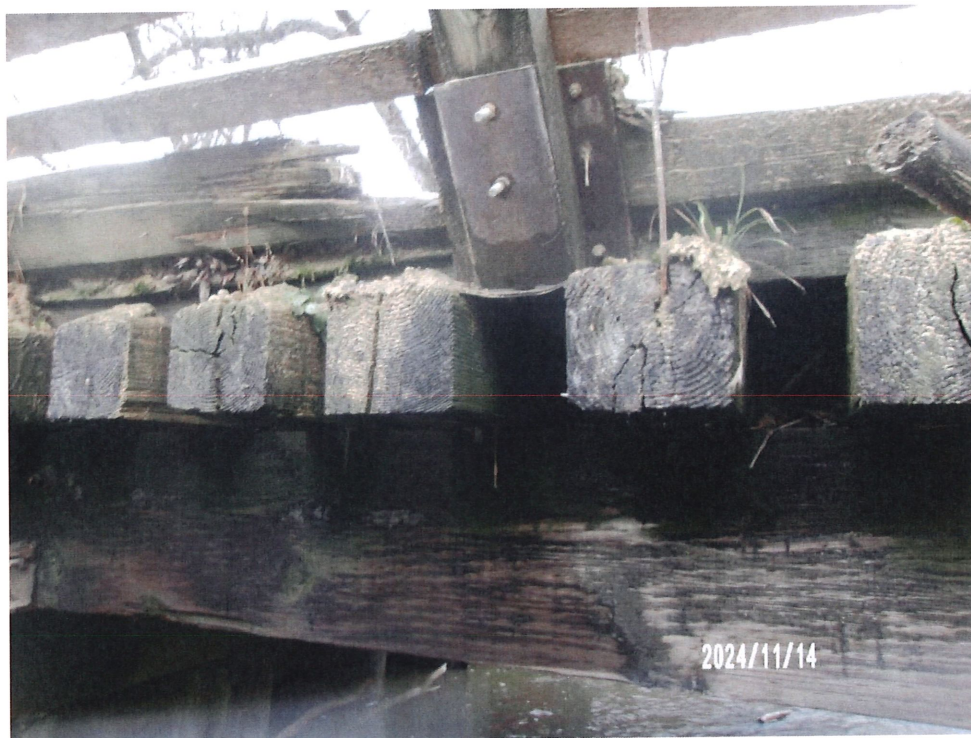
Figure 8: Typical Floor Beam Splitting
