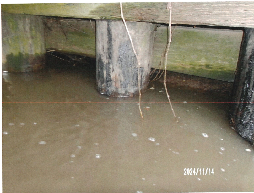
Figure 12: Undermining at North Abutment
