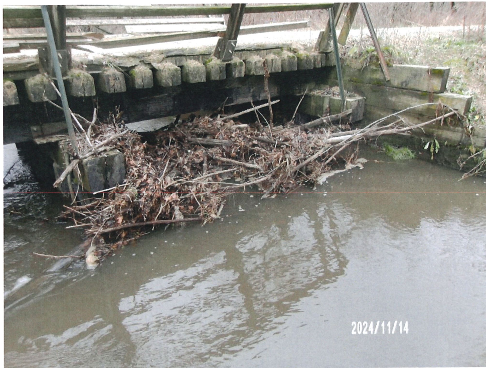
Figure 14: Debris at Upstream side
