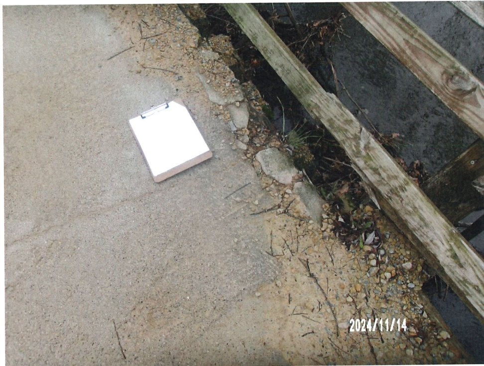
Figure 7: Deck Edge Starting to Spall Off
