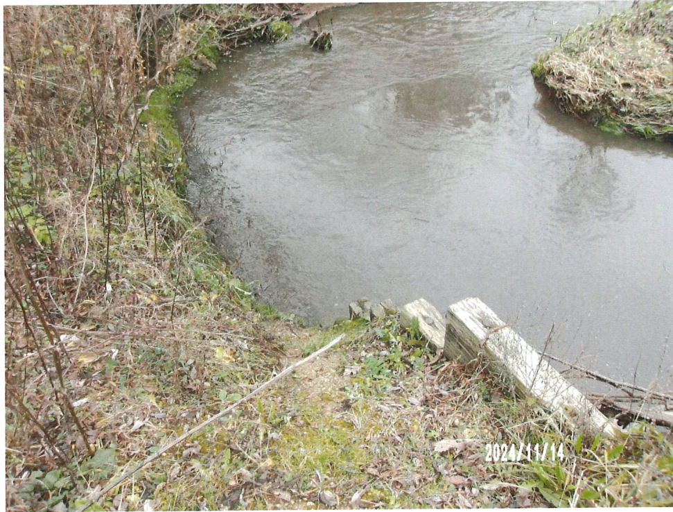
Figure 13: Stream Migrating Behind South Abutment
