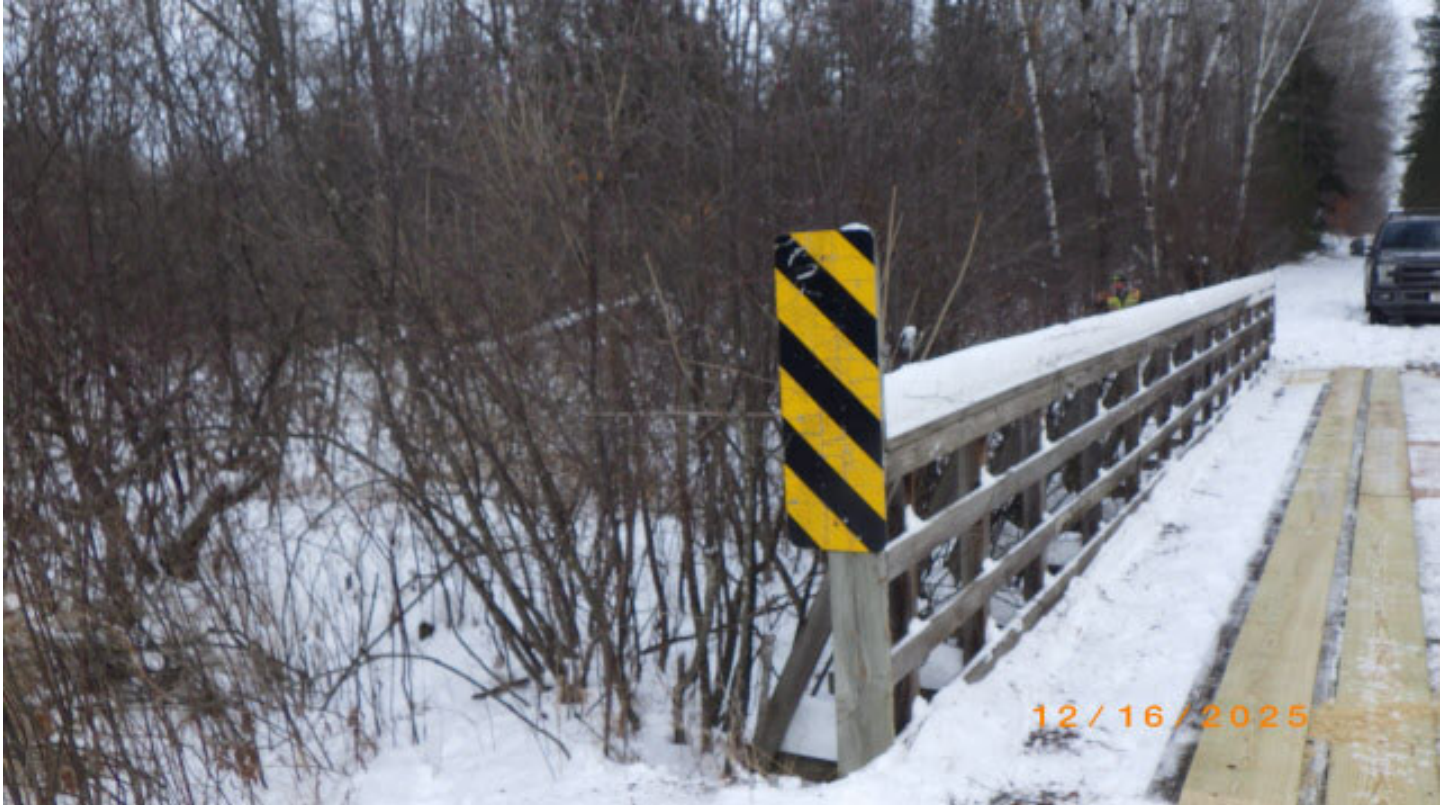
NW object marker, CS3 cracked
