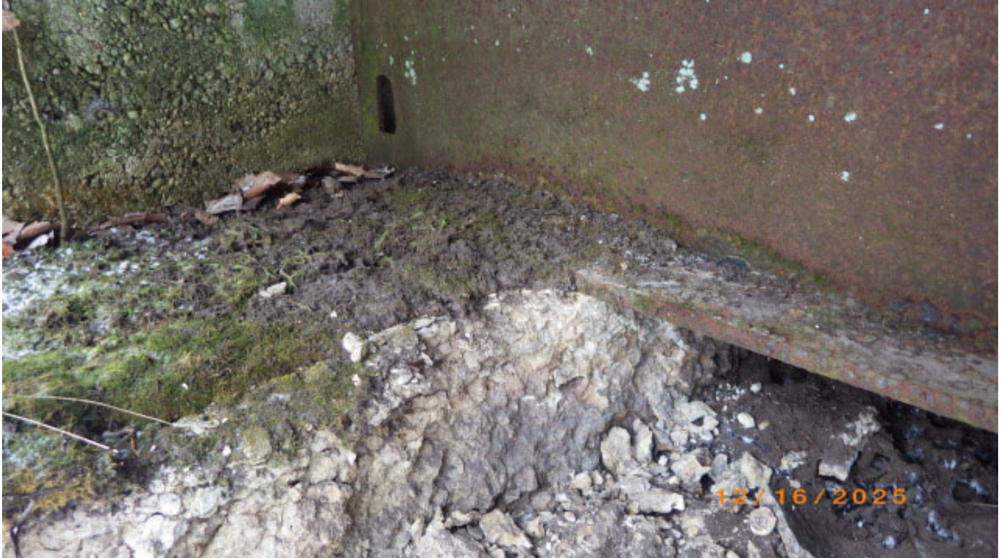
NE sill, CS4 spalling. Still good bearing for girder.
