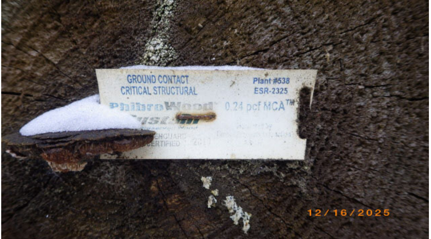
Treated wood tag, MCA treatment failed
