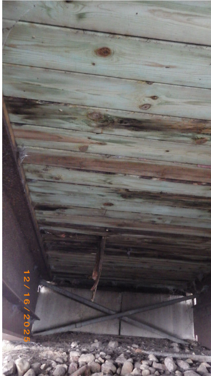
CS4 deck decay / partial failure
