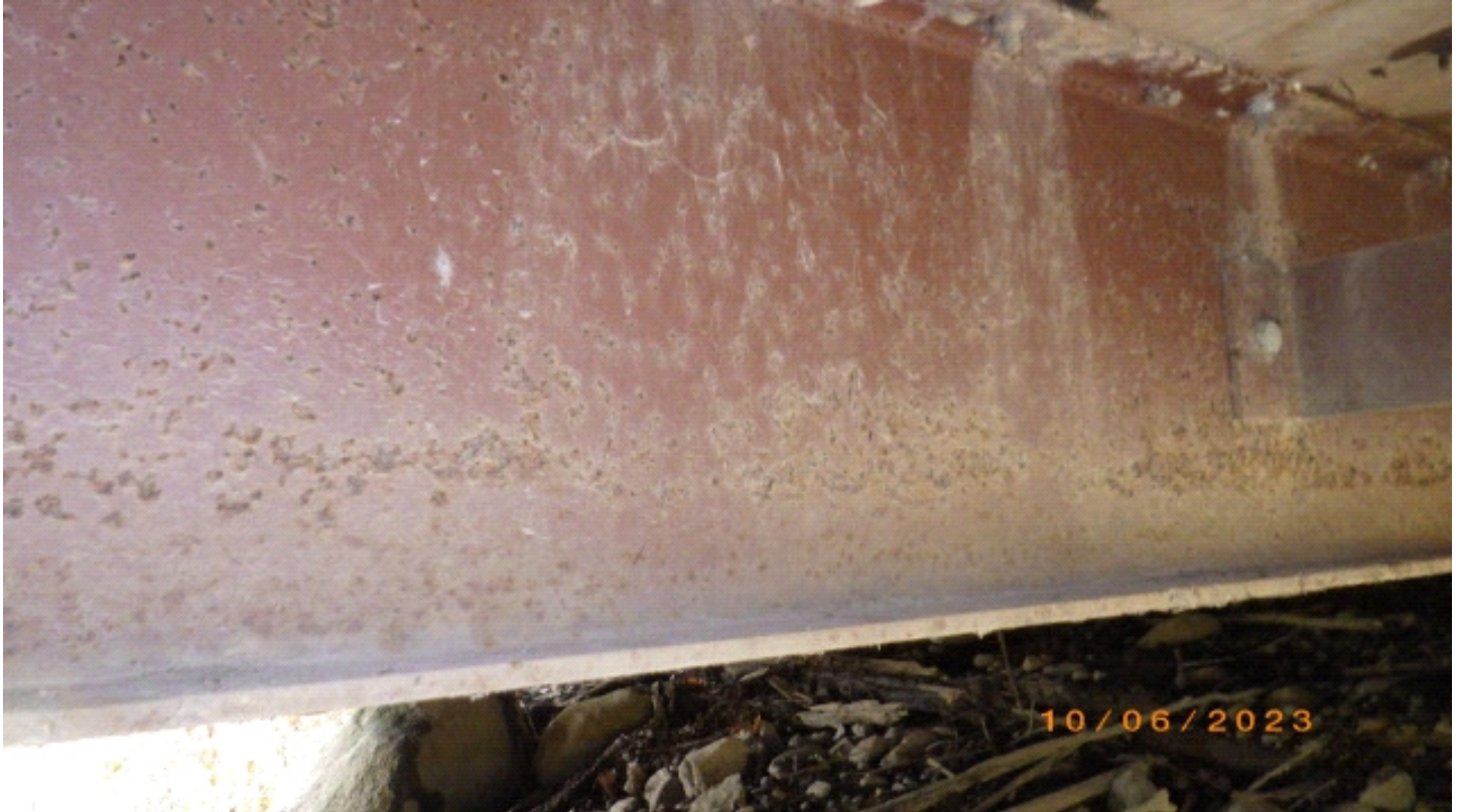
CS2 corrosion, typ.
