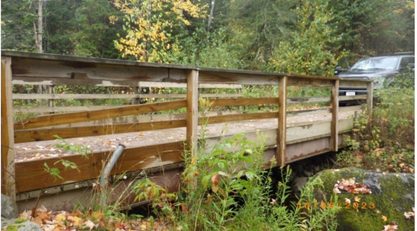
Looking West, damaged railing.
