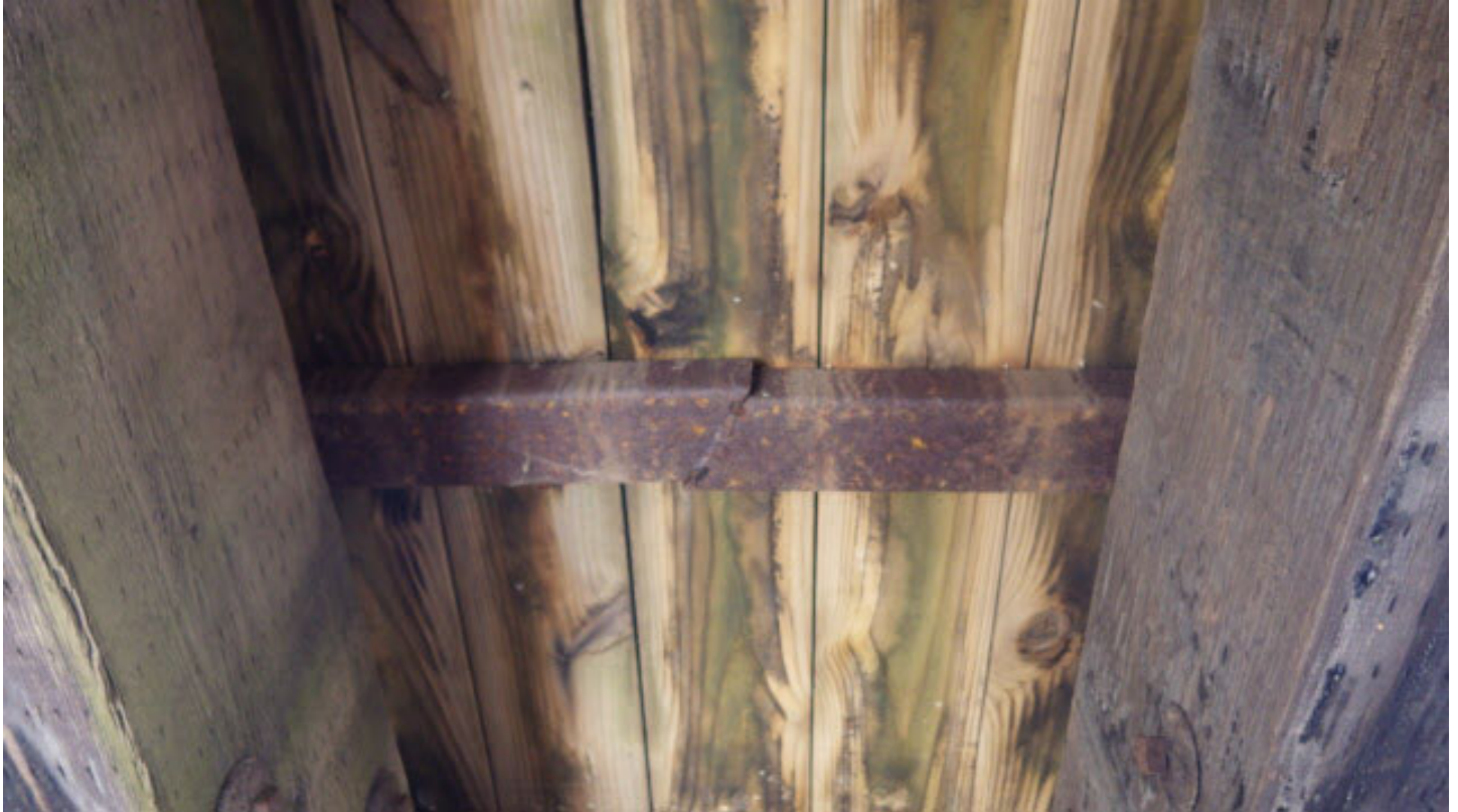
Floor beam in center of span 4 poorly spliced, moderate rust with no section loss
