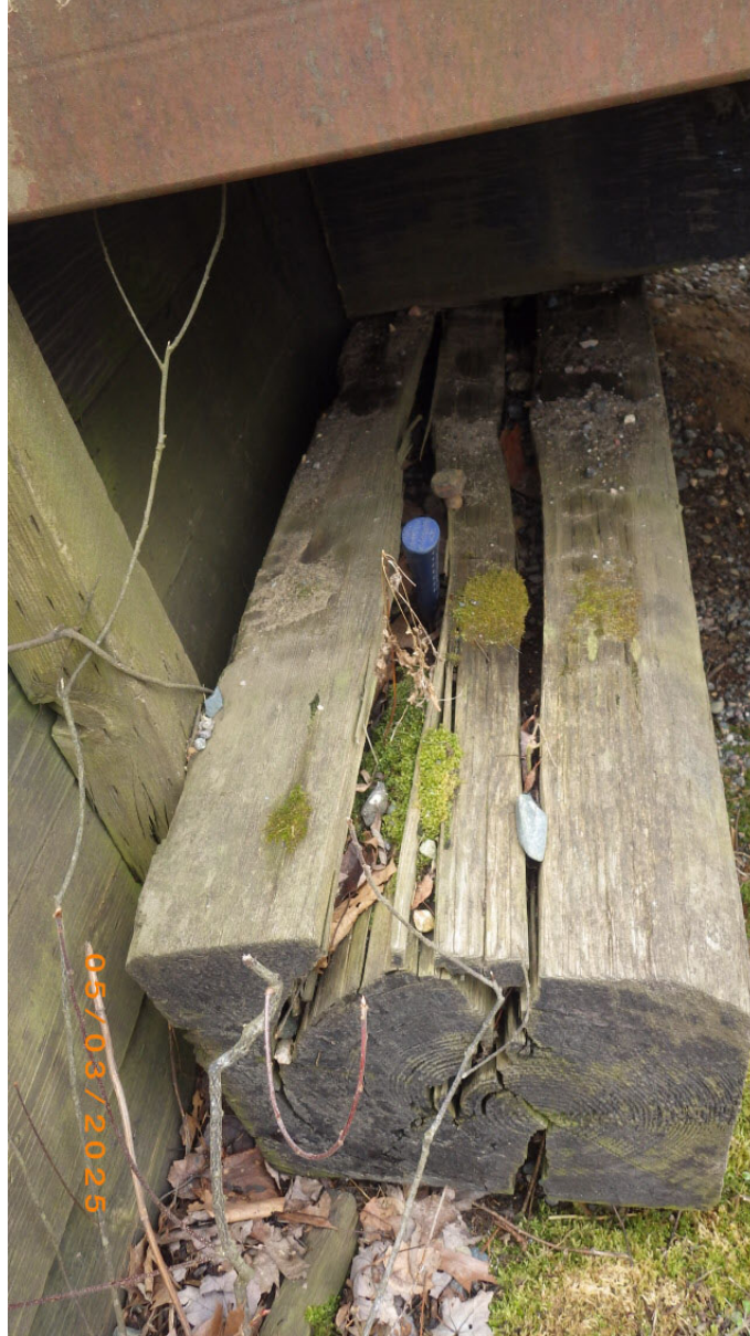
South abutment cap rotten / crushing
