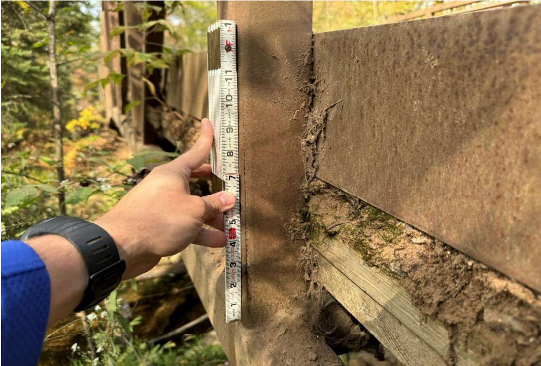
Closeup of L1 crack
