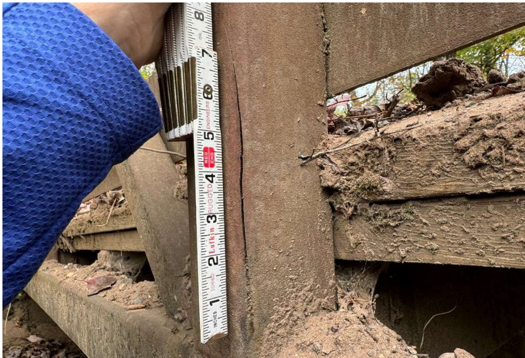
L6 panel point crack in vert
