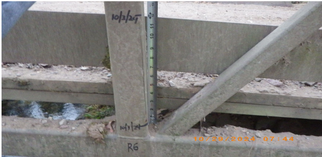
R6 vertical crack
