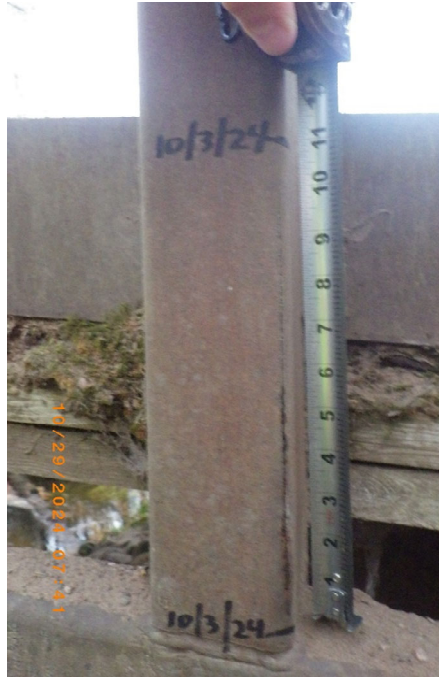
L1 Vertical Crack
