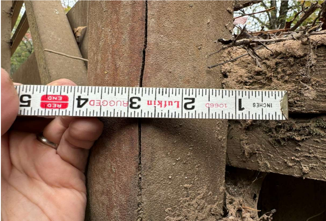
Another view of crack width at L6
