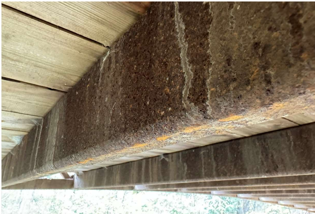
Typical FB condition
