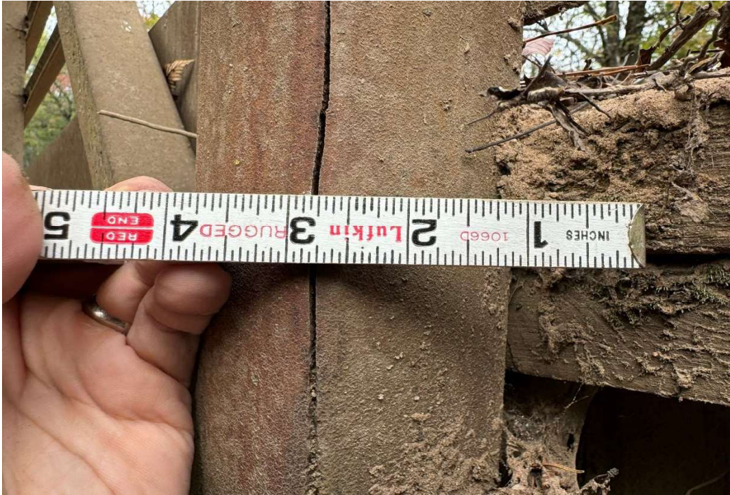
Another view of crack width at L6
