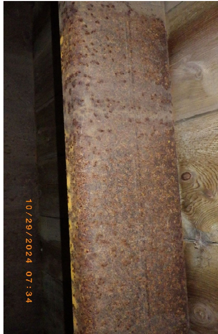
Typical rust on floor beams
