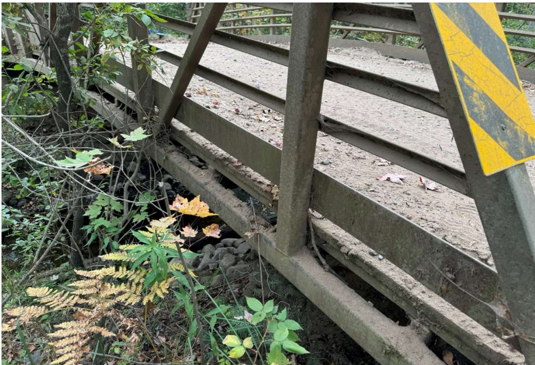
Toward R6 crack from NE quad
