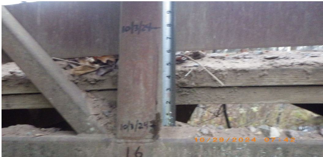
L6 vertical crack
