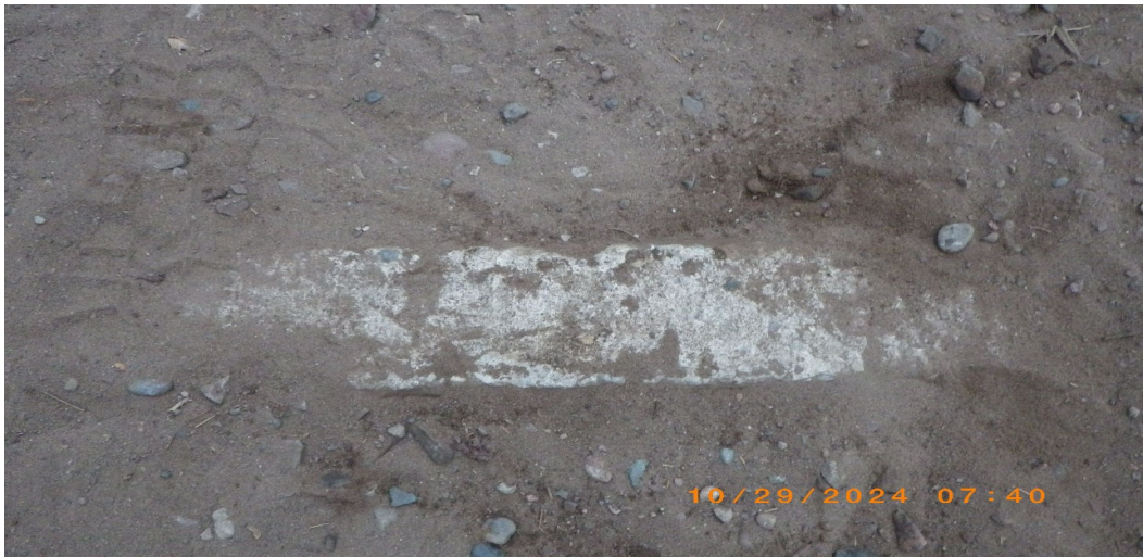
Backwall abasion where visible (SE quad)
