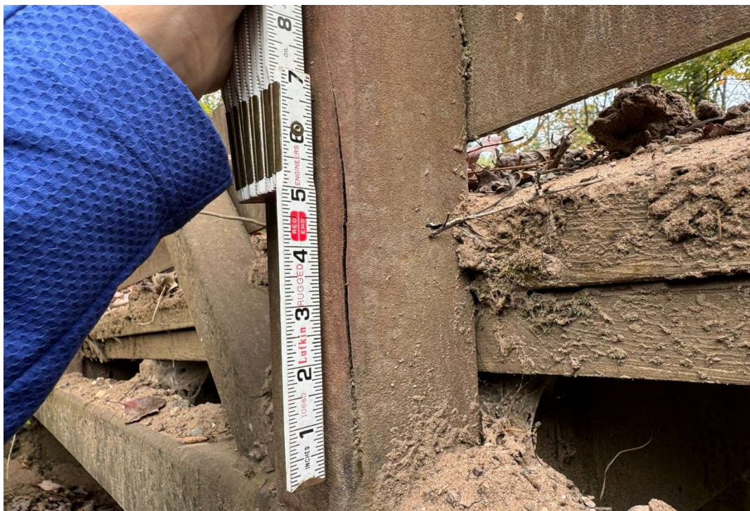
L6 panel point crack in vert
