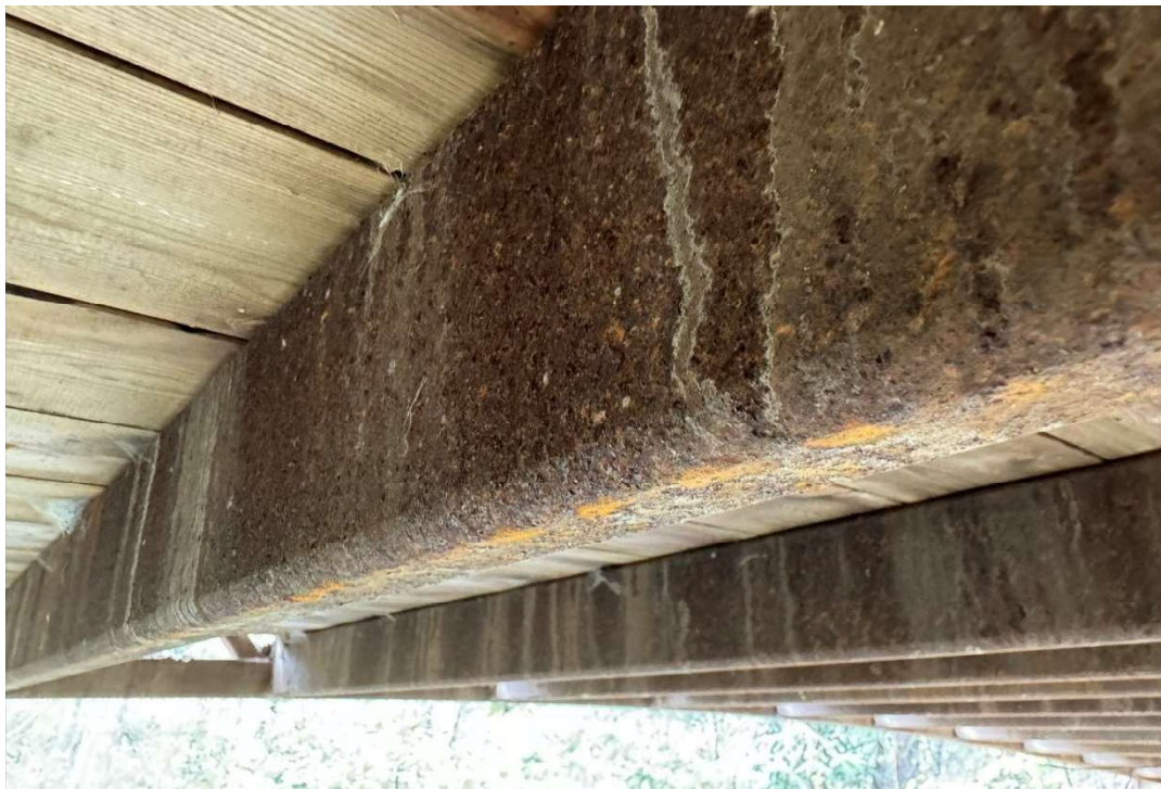
Typical FB condition
