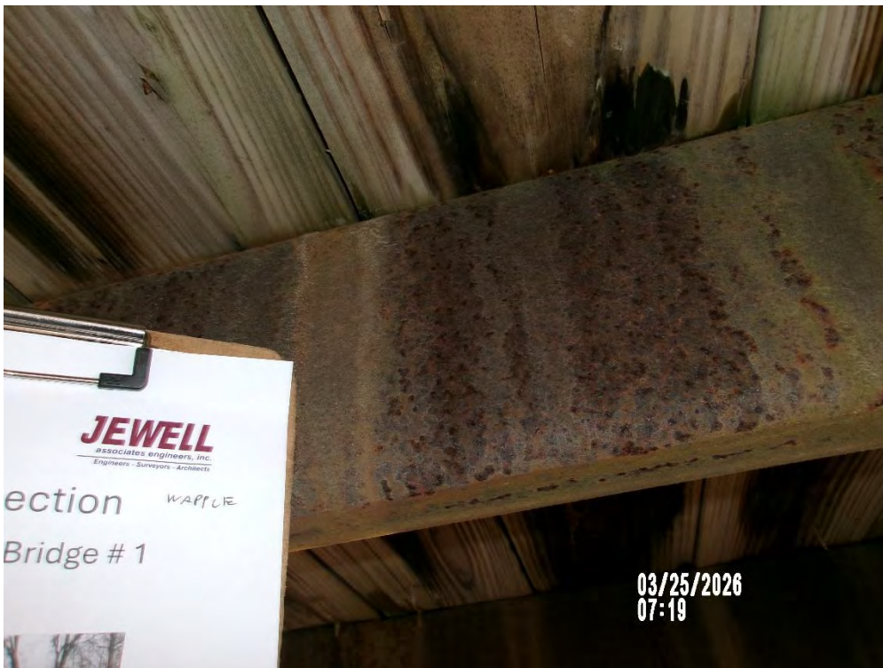
Figure 12: Worst case floor beam condition
