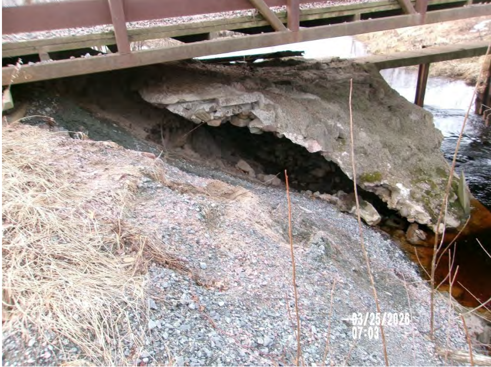
Figure 9: East slope protection undermining
