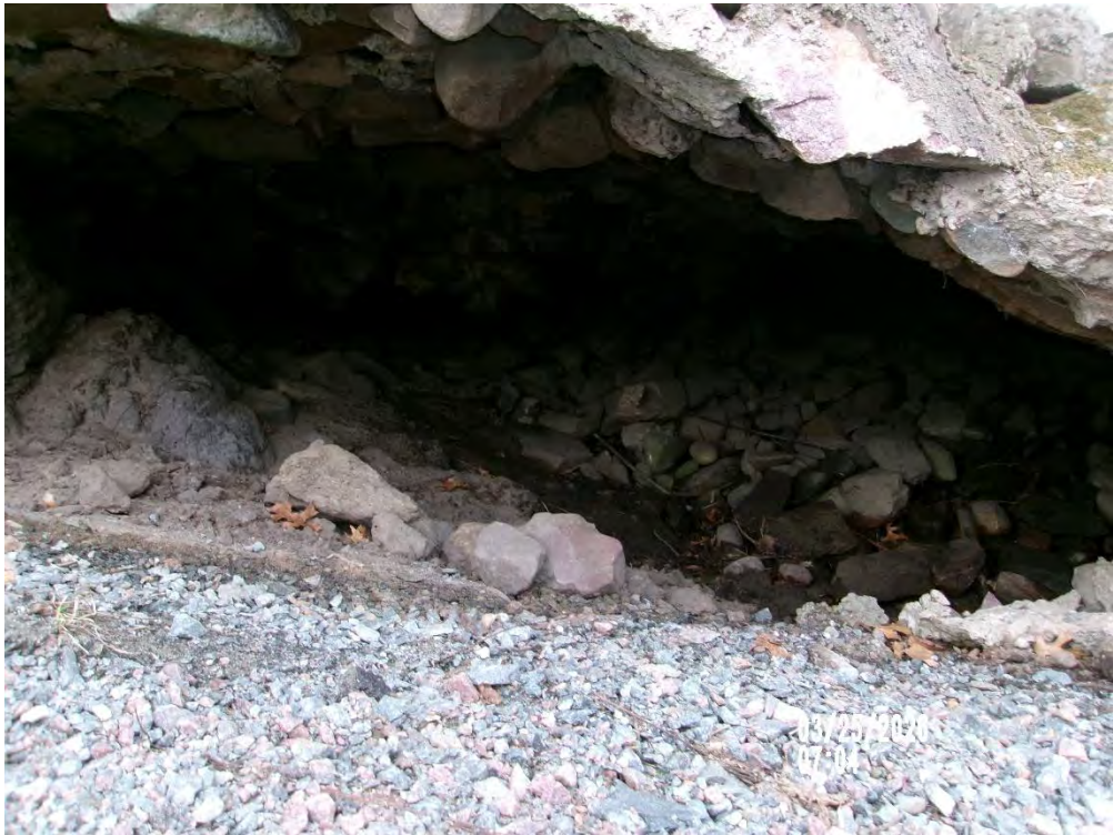
Figure 10: East slope protection undermining
