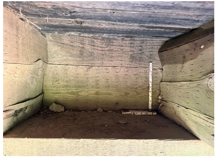
Photo 8 – Beams Crushing Over South Abutment.
