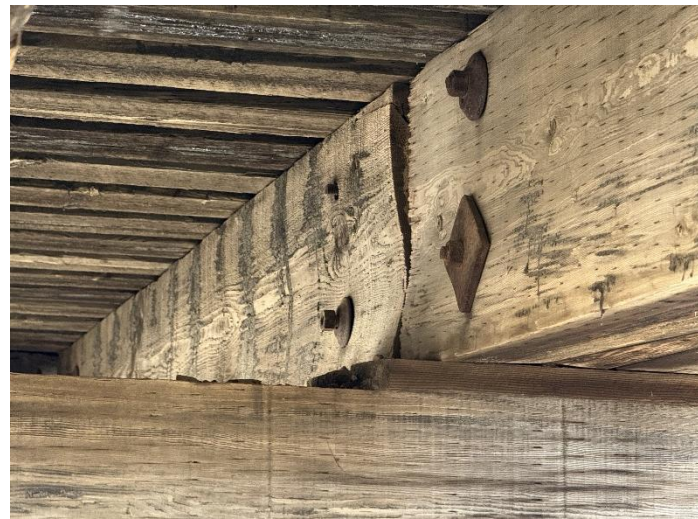
Photo 35 – N. Beam-S. Face Over Pier W5.
