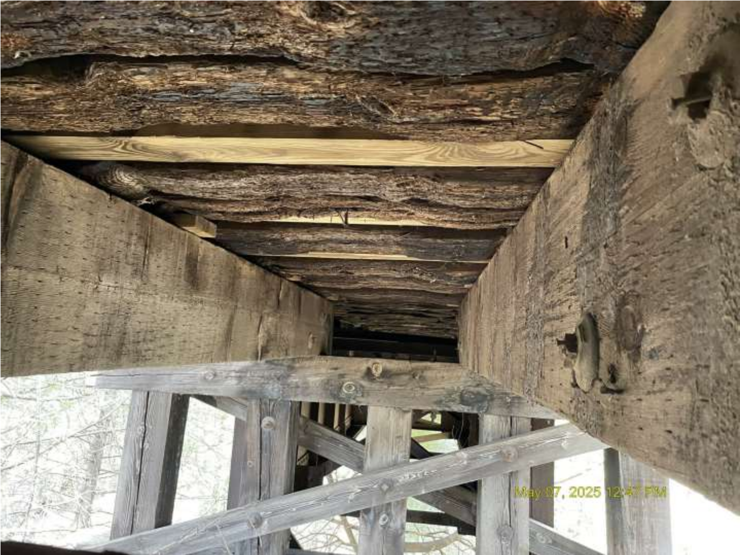
Looking (south) at rotted 8" x 8" RR ties
