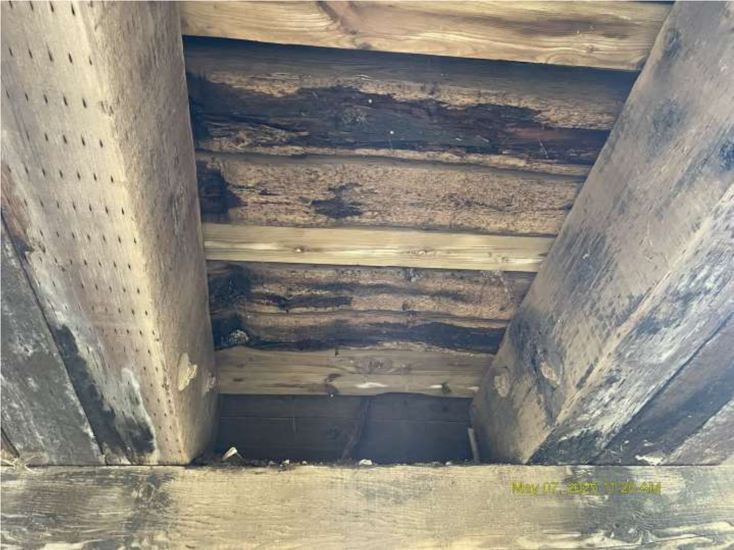
South end of bridge – rotted 8” x 8” RR ties
