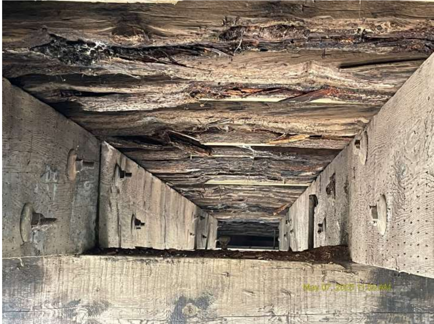
North end of bridge looking south – rotted 8” x 8” RR ties
