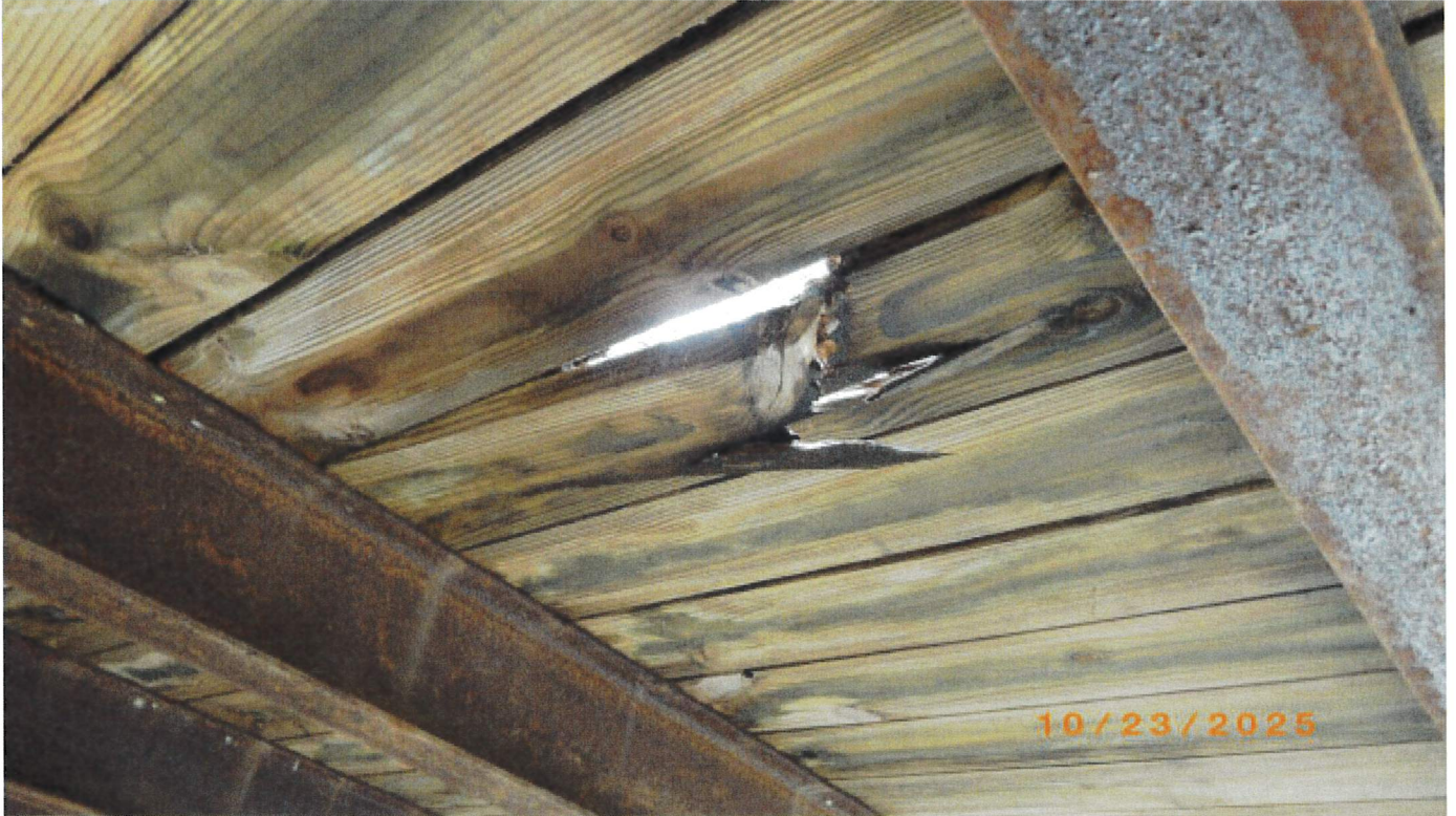
Hole through decking from below.
