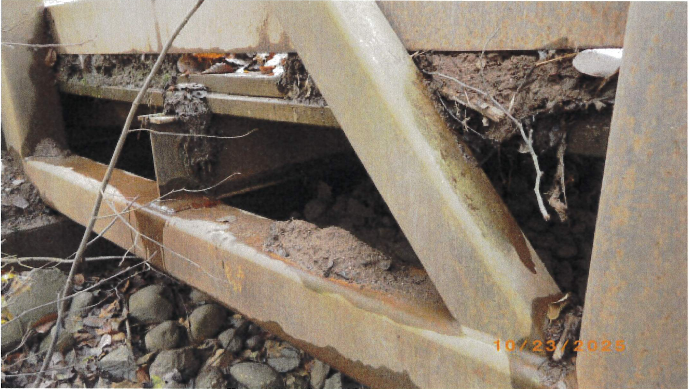
Sand on low chord ends
