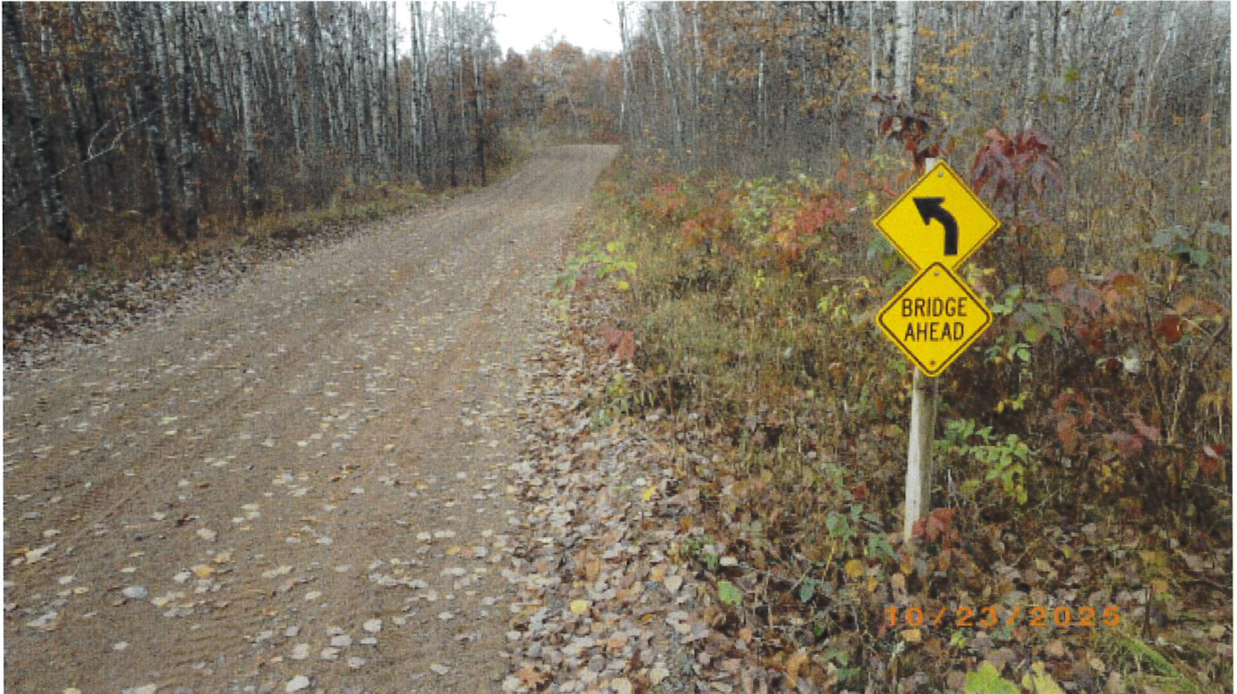
East bridge ahead sign, CS2 map cracked
