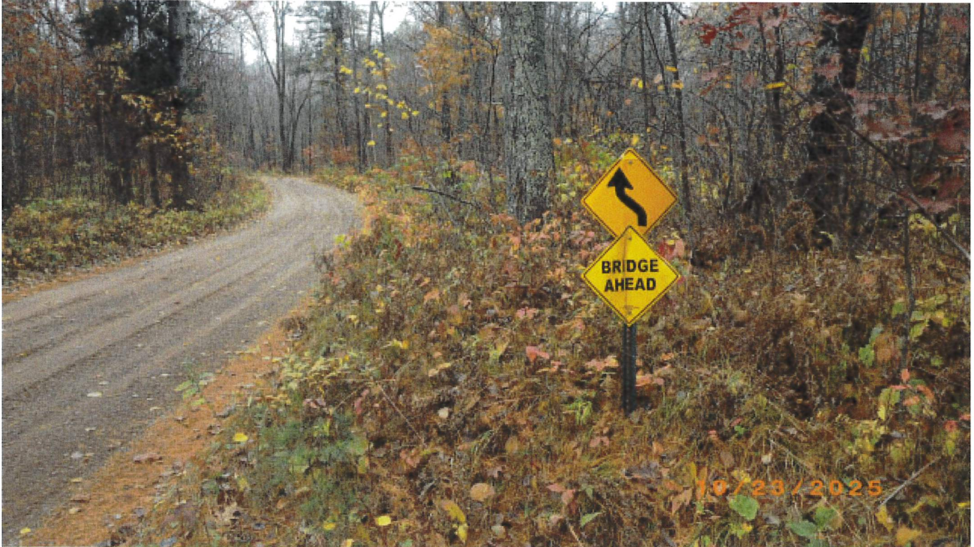
South bridge ahead sign, CS3 damage
