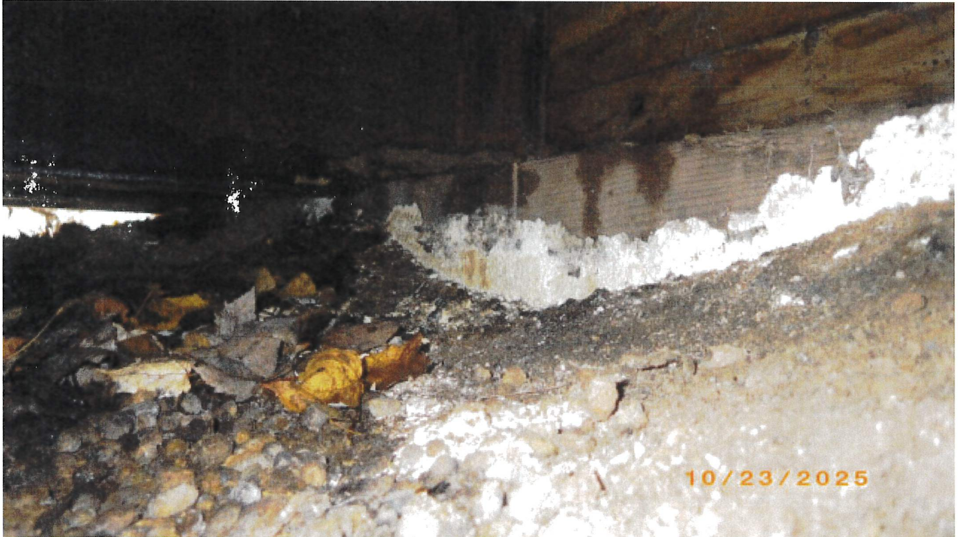
North sill white rot
