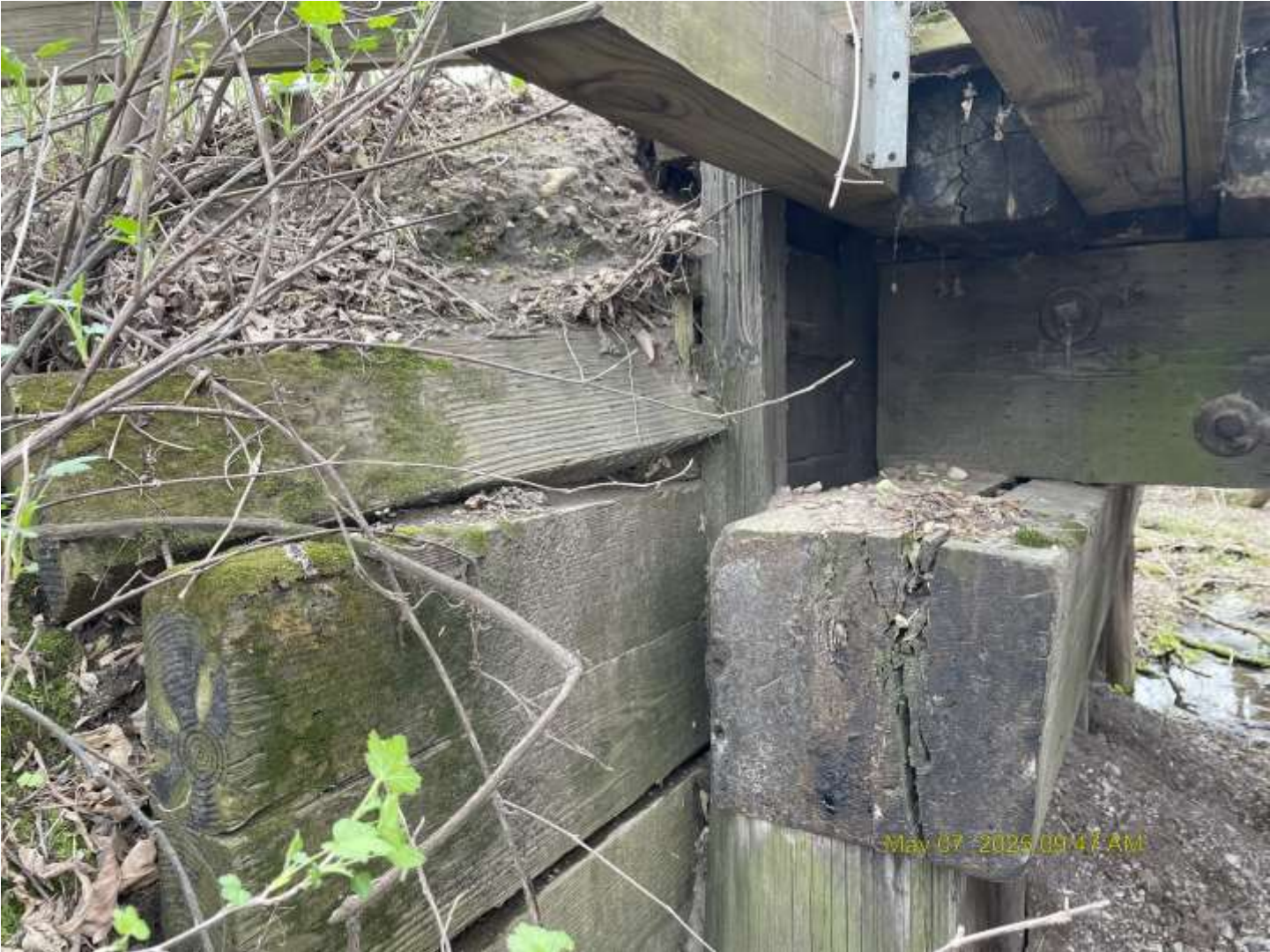
NE abutment wall failing
