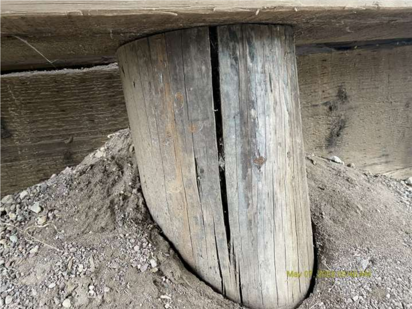
East center piling large split
