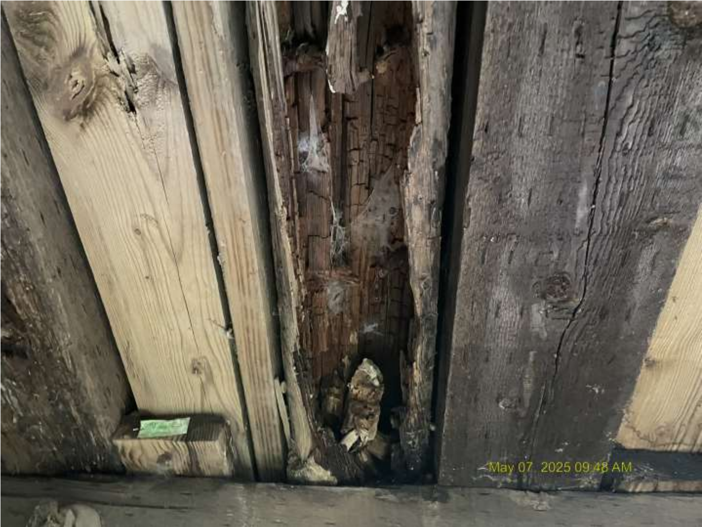
Underside RR ties rotted
