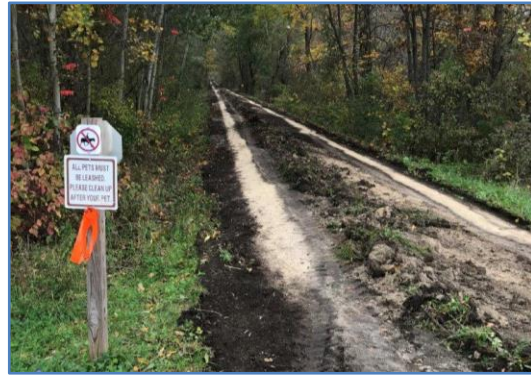
2. A small road grader was used to remove organic material from trail edges
