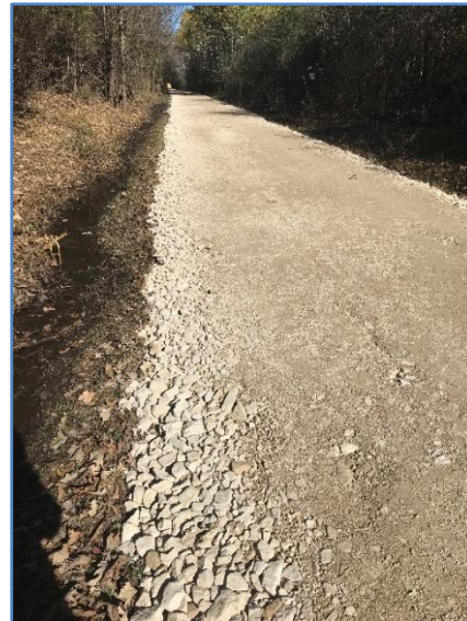
4. After re-surfacing with a six-inch compacted course of three-inch minus stone laid on the regraded trail. The original trail screenings below were still white and clean.
