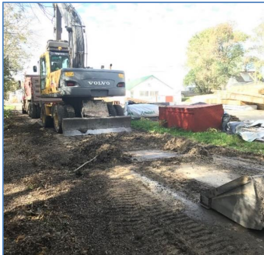
3. Equipment used to clean up and remove windrowed organic material: skid steer (bucket shown in the lower right), a small rubber tired backhoe, and a tri-axle dump truck.
