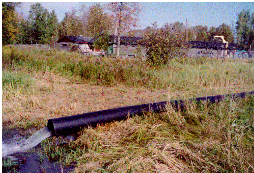
Salmon Stamp Funds Helped Pay for a Pipeline Has Been Installed to Increase Water Flow Through Strawberry Creek Weir
